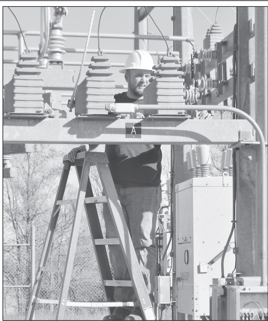
SQUINTING IN THE SUN , Justin Byarlay of Mid-States Energy Works out of Salina surveyed part of the city's main electrical substation, which was being prepped Monday for installation of a refurbished transformer. - Herald staff photo by Stephanie DeCamp
