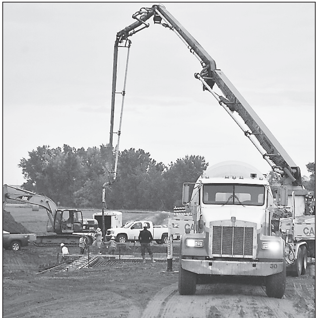
CONCRETE WAS POURED out of a revolving tank, into a pumper truck, up and out a spout, and then finally through a pipe that led to the forms of the new bridge 13 miles south of Oberlin and a mile west of U.S. 83. The bridge, poured last Tuesday, will likely be finished in the next few weeks. - Herald staff photo by Stephanie DeCamp
