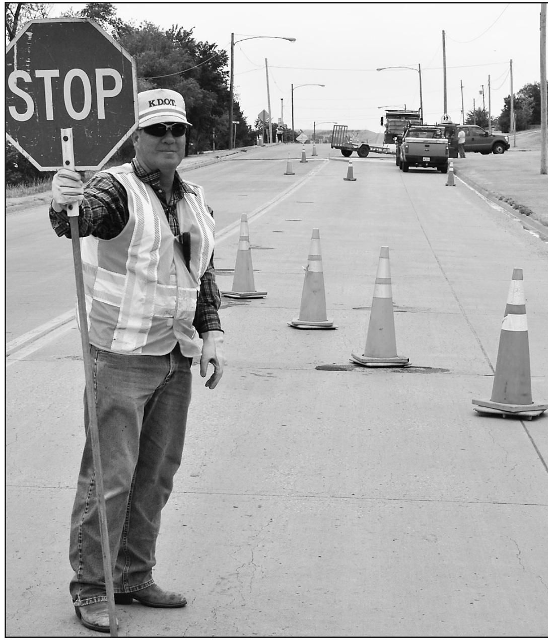
DAVE DEPPERSCHMIDT held up a stop sign for travelers on Tuesday as Kansas Department of Transportation workers repaired a buckle in the concrete of U.S. 83 near Elm Street in Oberlin.
