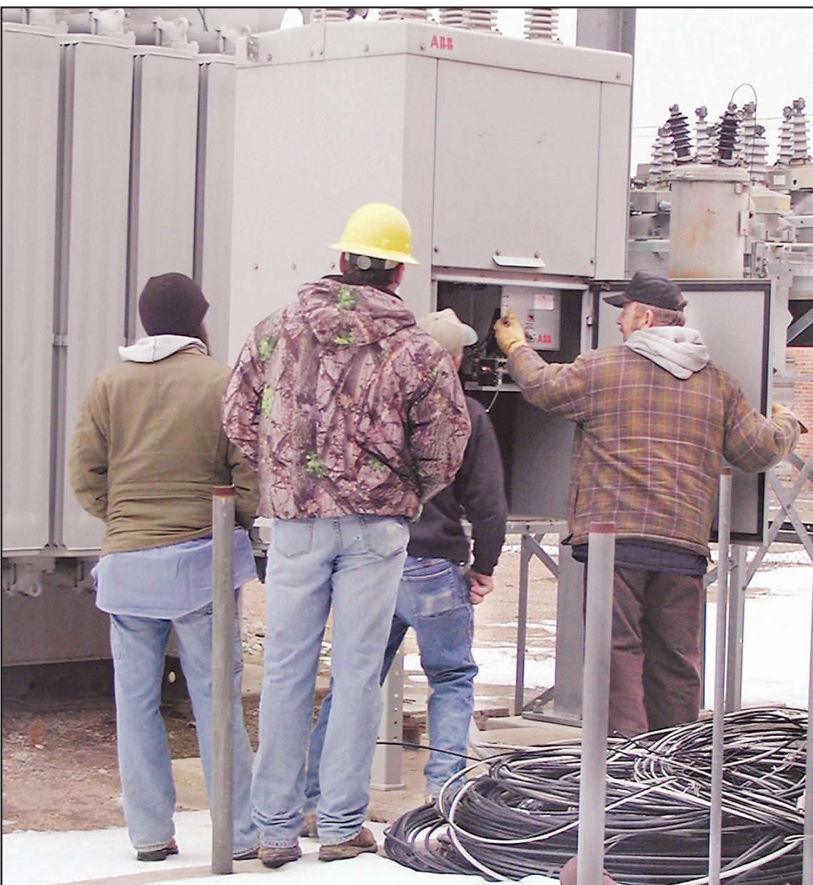
AT THE CITY POWER PLANT on Monday morning, Foreman Dan Castle (right) got things going so the entire town could have power. Other linemen from Oberlin, Sunflower Electric and Prairie Land Electric helped the city get power on after its main substation burned early Monday morning. — Herald staff photo by Brandi Diederich
