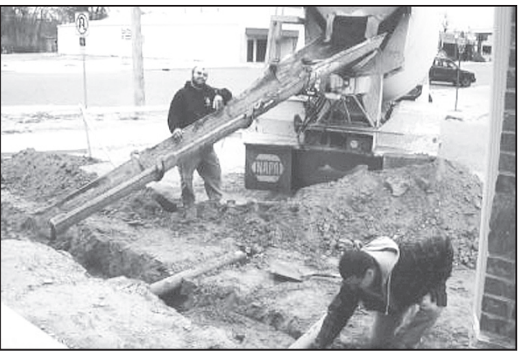
AN OBERLIN CONCRETE employee, Carl Stately (left) unloaded concrete for the new wall being built at the south side of the Oberlin Meal Site. Checking it out was owner Wayne Hackney. — Photo by Marie McKisson
