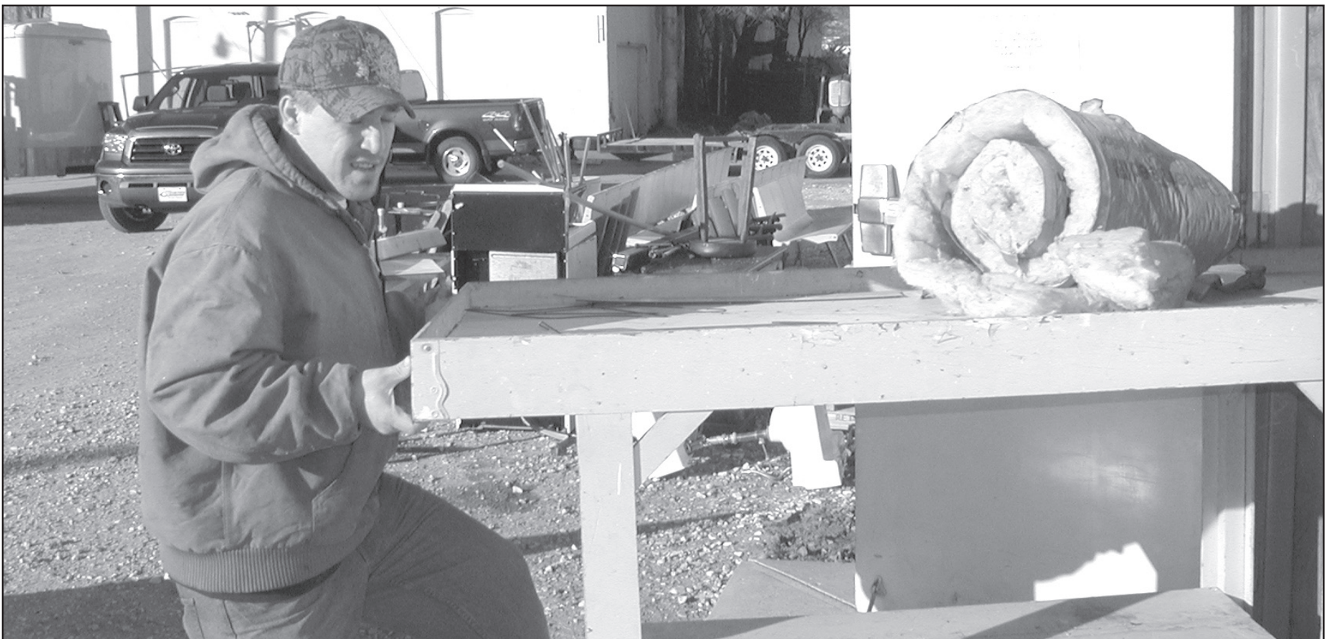
VOLUNTEER LEVI JONES FROM COLBY helped move tables and insulation out of the Golden Age Center building, which will be demolished to make room for a new senior center, theater, bowling alley complex, which will be built on the site.
