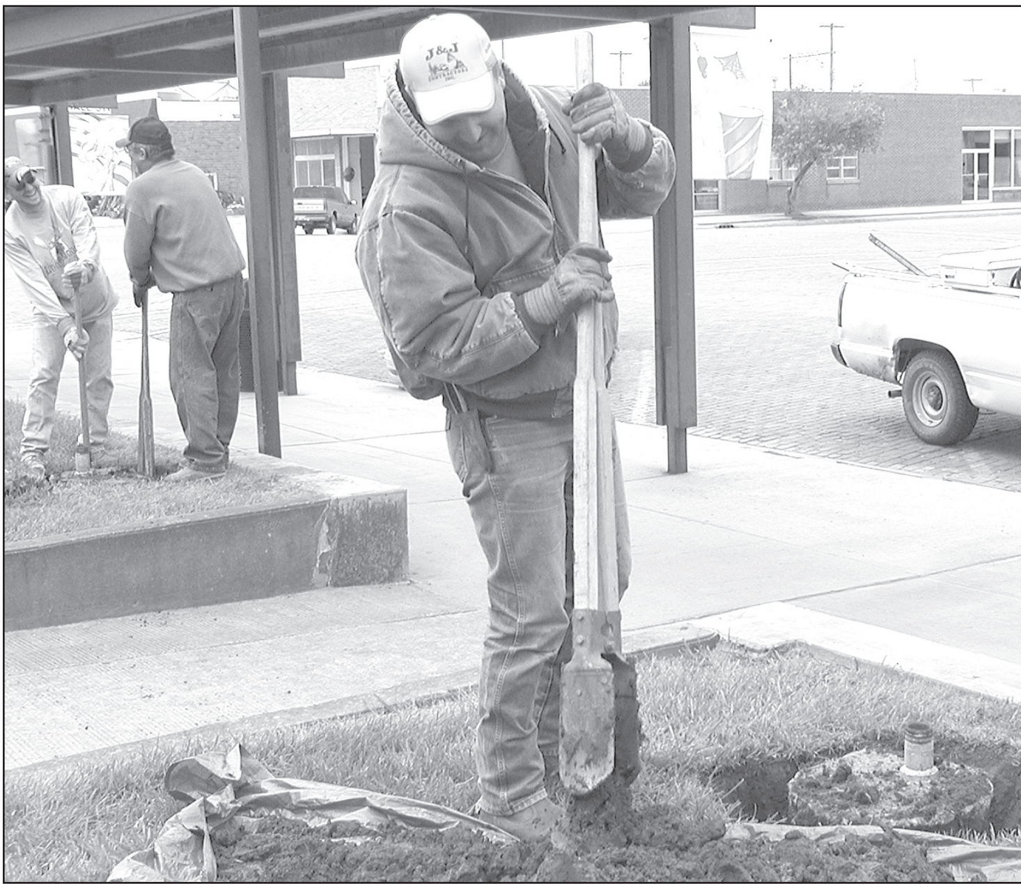
ON THE WEST SIDE of the Decatur County courthouse, Seth Lohofener used a post-hole digger to remove dirt from around the concrete bases that formerly held the flag poles, while two of his colleagues worked on the other side. The flag poles are being moved to the front, or south, side of the courthouse. — Herald staff photo by Kimberly Davis
