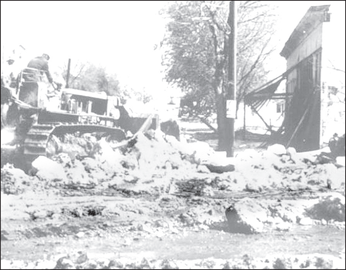
ICE WAS BULLDOZED into piles against the background of the sagging awning in front of the Farmers Union building in Selden. Workmen labored all day to clear hail from the streets and debris from collapsed sections of buildings.
