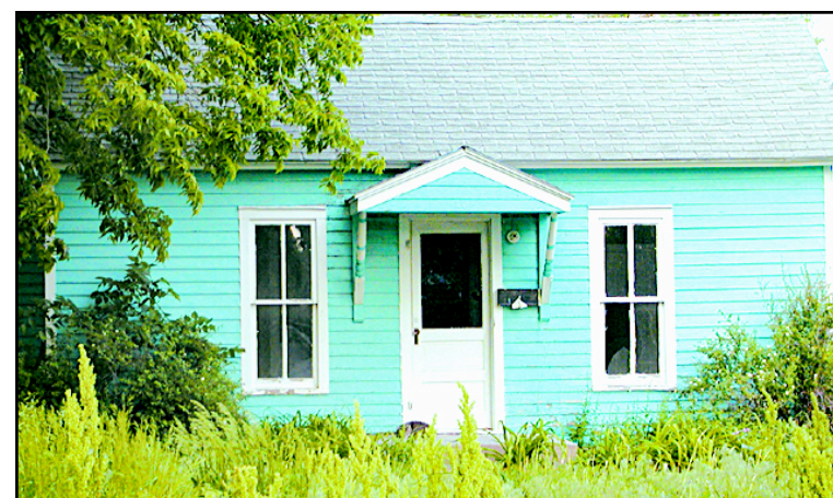
THE CITY received a petition about this house at 107 N. East Avenue to declare it abandoned. — Herald staff photo by Kim Davis
