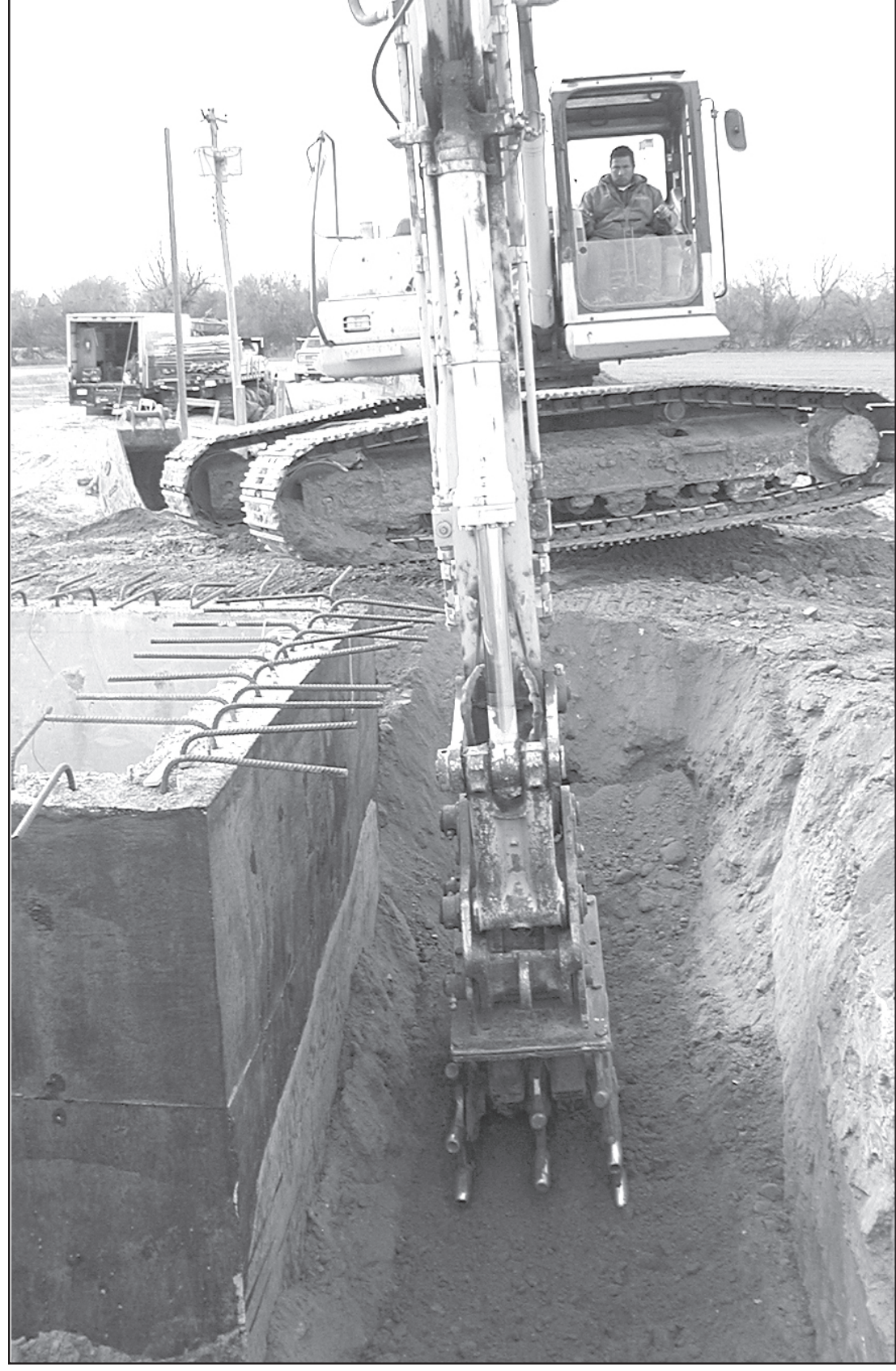
A CREW WORKED at the city's new waste water treatment plant on Friday afternoon. One of the men with Midlands Contracting used a backhoe to move dirt out from the sides of the new lift station on the north side of the creek. — Herald staff photo by Kimberly Davis
