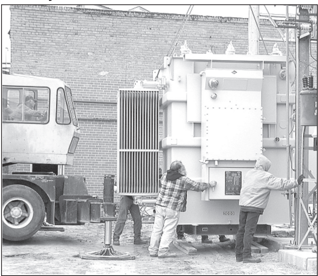
AT THE CITY POWER PLANT last Tuesday, a crew from Midstates Contractors of Salina, Solomon Transformer Co. out of Solomon and a Hixson Construction crane from McCook helped put in the new transformer. The city crew generated power while the transformer was installed and hooked up. — Herald staff photo by Kimberly Davis
