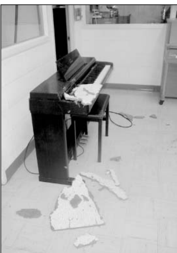
A LEAKY ROOF caused extensive damage to a clavivova and papers on Band Teacher Deanne Spanier's desk.
