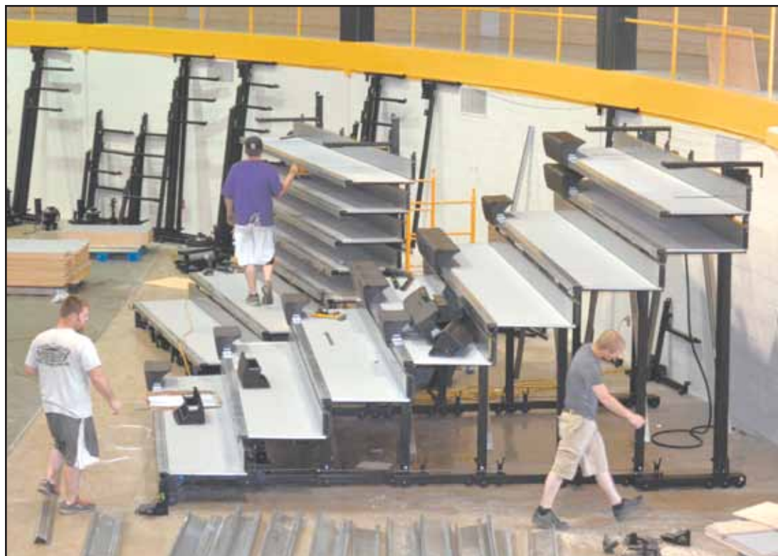
New south-side bleachers are currently being installed at Max Jones Fieldhouse. When finished the Max will completely have new bleachers. The money has been raised by the Cowboy Booster Club. The ceiling at the Max has also been painted. Photo by Pat Schiefen/The Goodland Star-News
