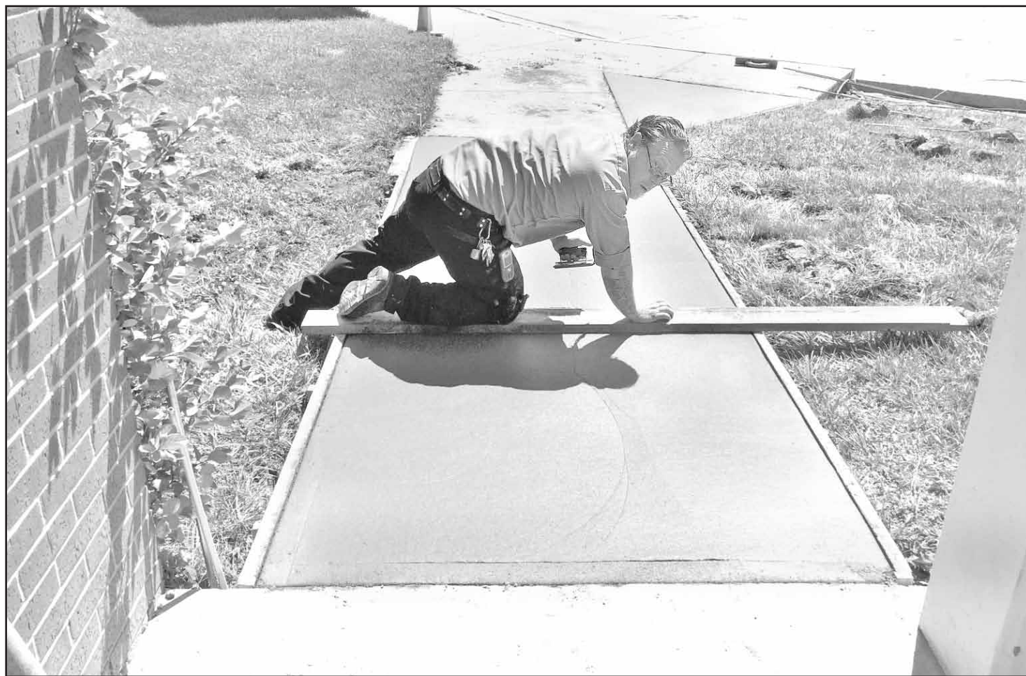
Nick Arnold recently worked on replacement sidewalks at the Goodland Regional Medical Center as part of the hospital's continuing efforts to meet Americans With Disabilities Act guidelines. Photo by Mark Riley/Goodland Regional Medical Center
