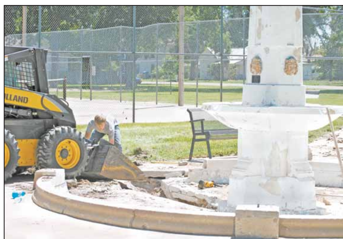
New work is being done to restore the Victory Memorial Fountain at Chambers Park. The goal is to bring the fountain back to life with functioning water plumbing. The fountain — which was originally a World War I memorial — was completed in 1930. Photo by Kevin Bottrell/The Goodland Star-News
