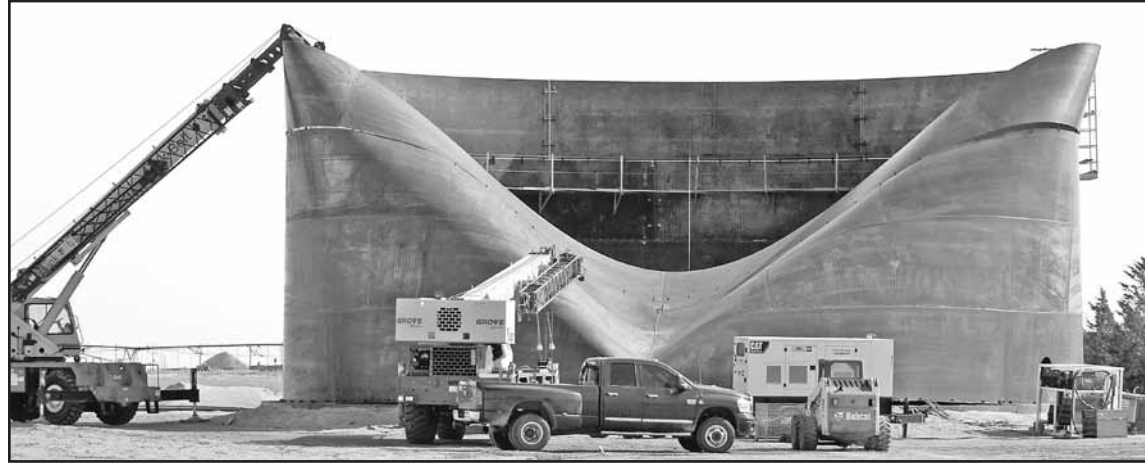
This half-finished fertilizer silo at Crop Production Services was bent inward by a gust of wind on Thursday. Crews worked over the weekend to repair the damage.
