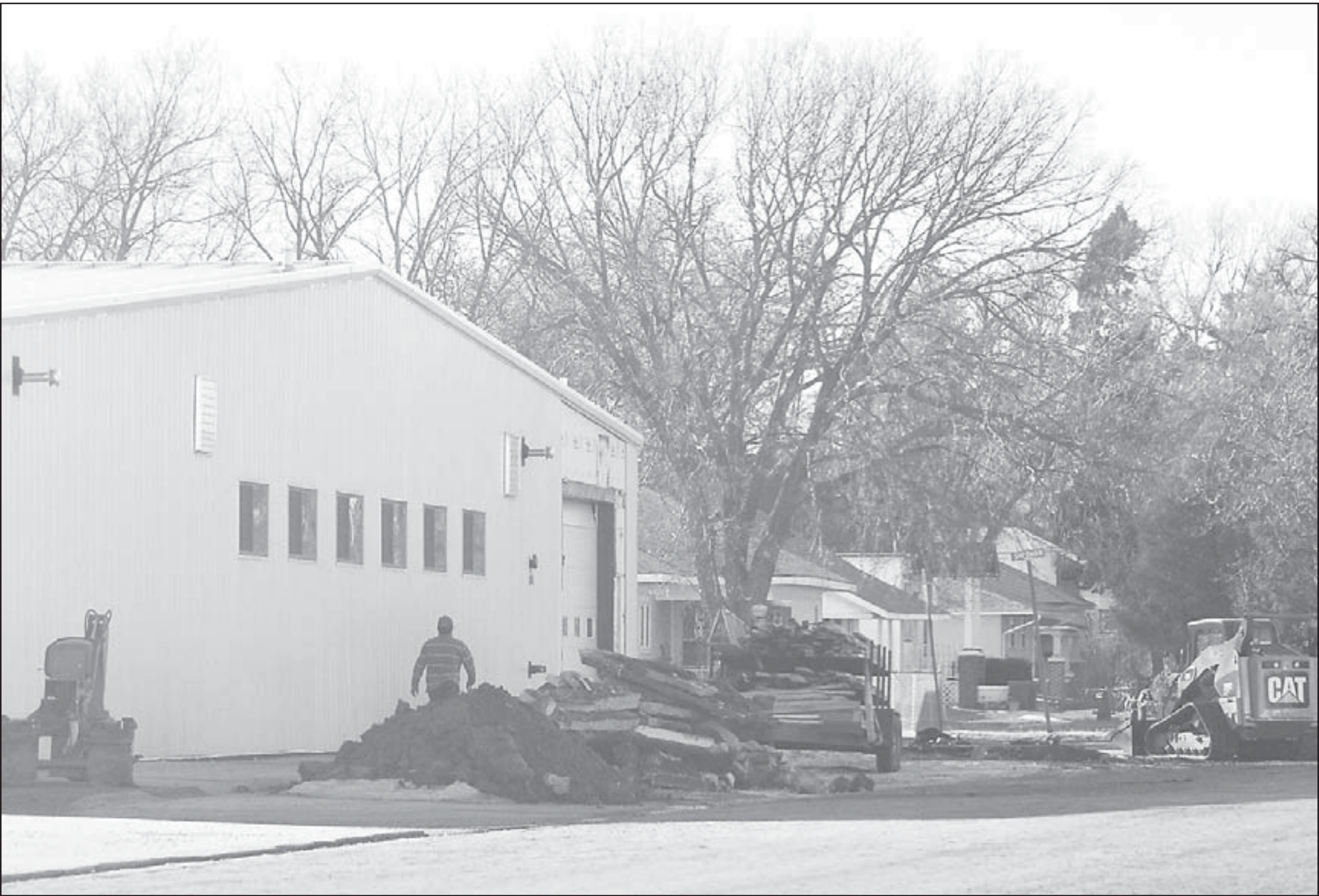
Work has begun on the new fire and ambulance station. The Wolak building, which at various times has been a supermarket and a manufacturing plant, will be remodeled into a joint station for the
