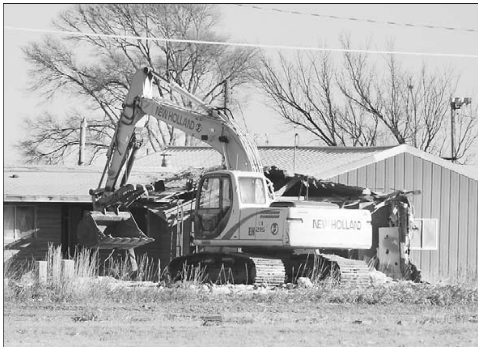
Crews were working on demolishing a building at Motel 7 on U.S. 24 last week.
