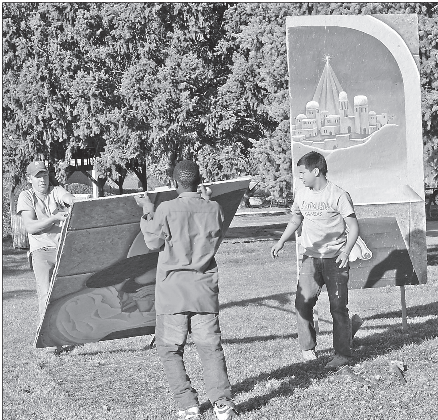
Students from the carpentry class at Northwest Kansas Technical College worked on erecting the Nativity Scene that is put up around Goodland Regional Medical Center. The three artists who created it were Connie Hatcher, Jeanette Foust and the late Max-
