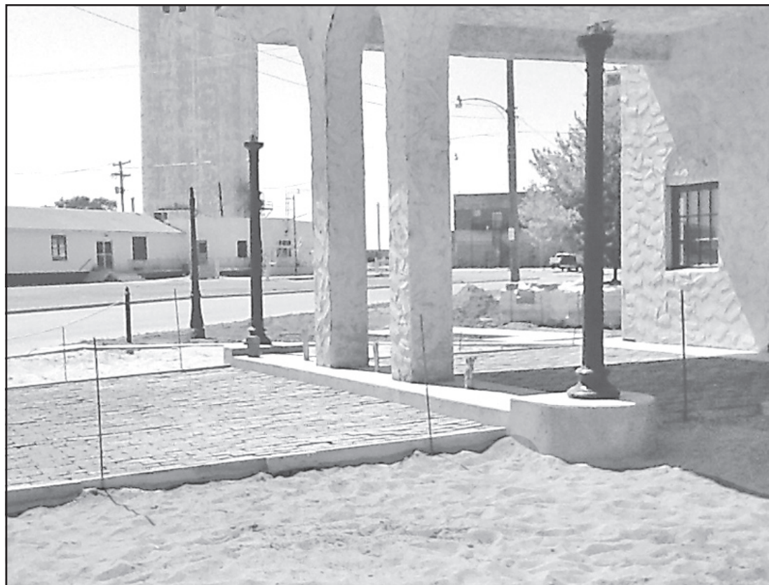
Work has been ongoing to fix up the old gas station owned by Rod Cooper that was moved to 17th Street and Clark Avenue and the surrounding landscape. The latest work is a brick driveway using old bricks from Main Avenue.
