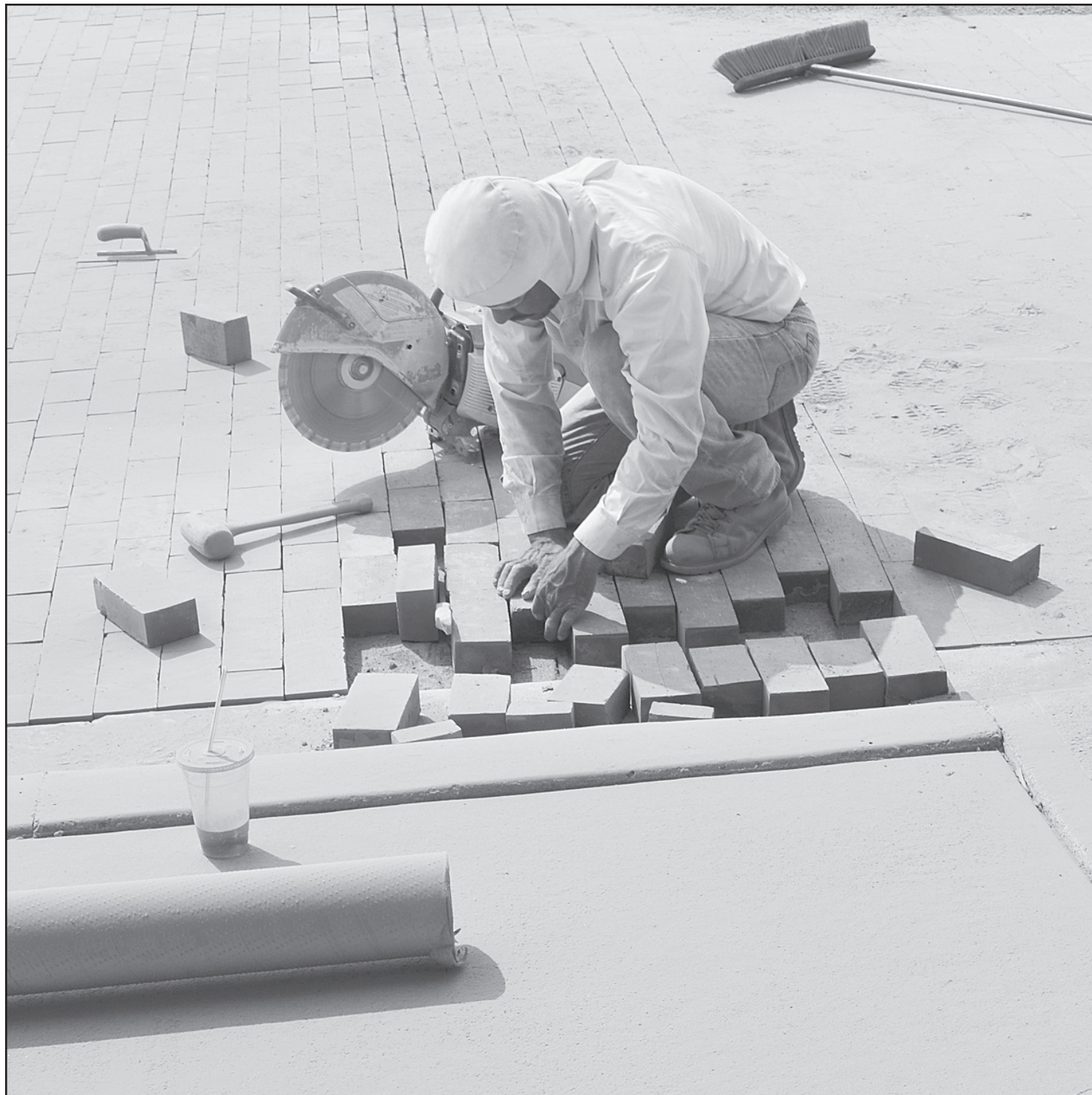
One of the brick layers worked on getting the last few bricks to fit in the brick replacement project on Main Avenue between 12th and 13th. All of work was done and even the stripes for parking painted before the first day of school on Monday. Photo by Pat Schiefen/The Goodland Star-News
