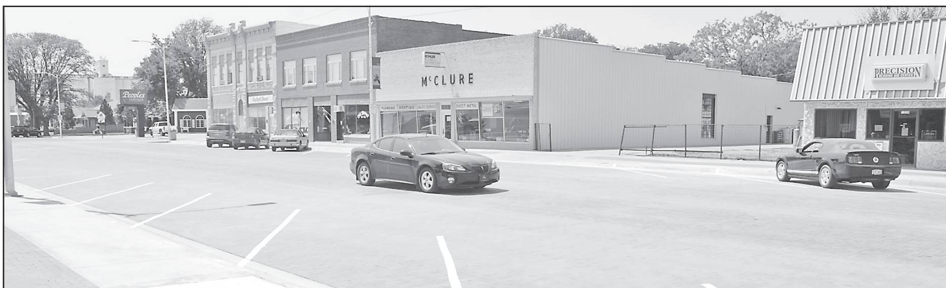
The long-awaited day when Main Avenue from 12th to 13th Streets would finally be reopened came on Friday, when contractors finished laying the last few bricks. The months long process to tear up the two blocks between 11th and 13th Streets began in May. The crews also laid new water pipes under the sidewalks and put brick over them for easy access. Photo by Kevin Bottrell/The Goodland Star-News
