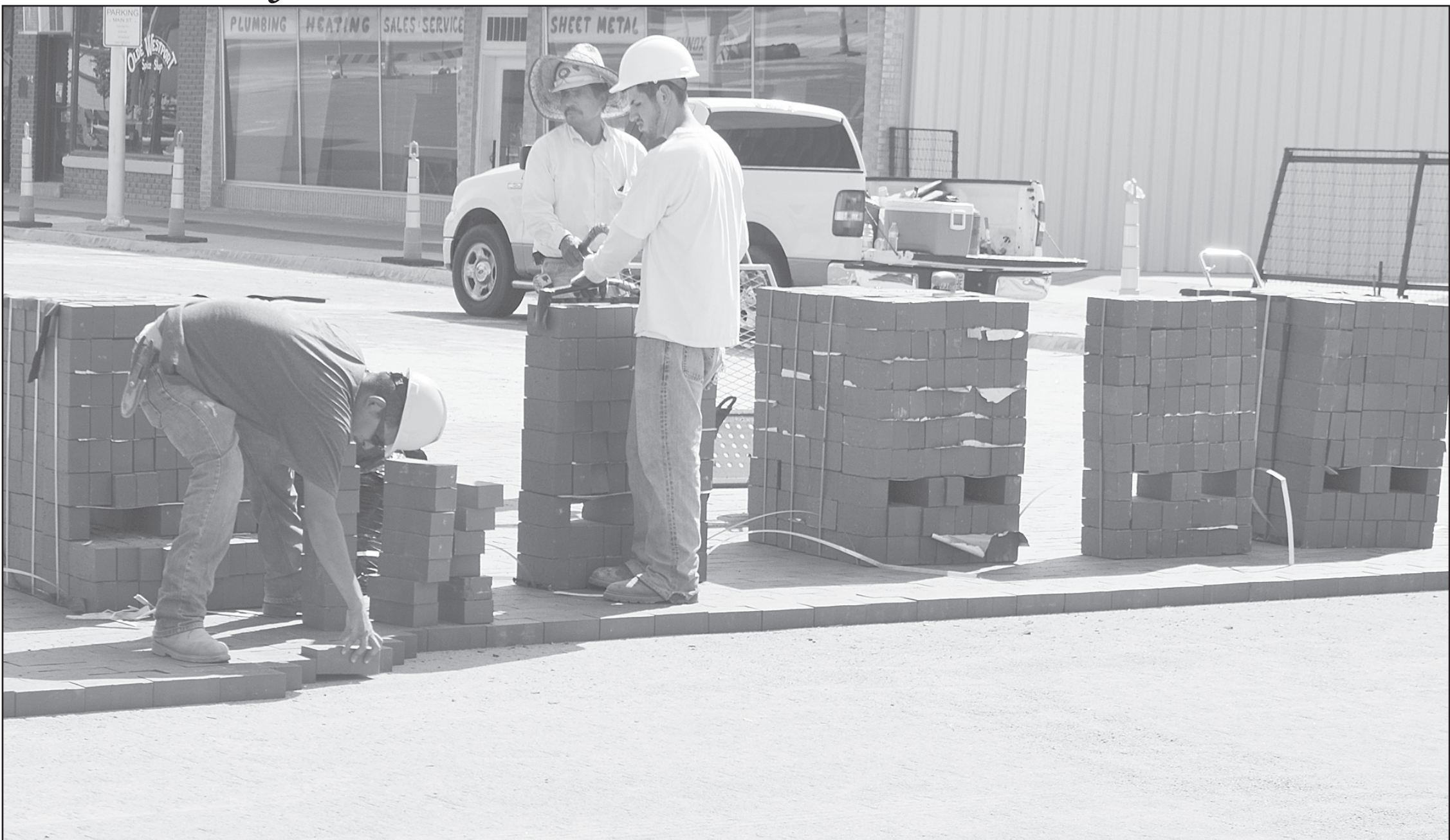
Brick layers working on the block between 12th and 13th on Main Avenue finished on Thursday. Bricks, water and sewer lines were replaced on the two blocks between 11th and 13th. The street had to be done before Flatlander Fall Festival the last weekend of September. Businesses on the street were anxious for the street to be done. Photo by Pat Schiefen/The Goodland Star-News
