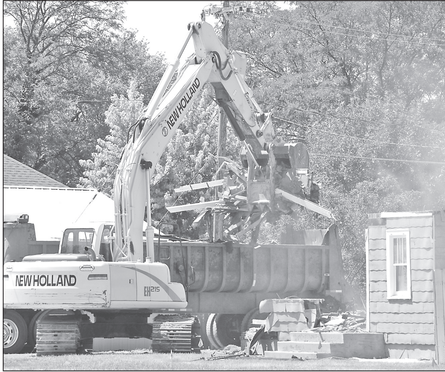
This small house on Caldwell Avenue was demolished over several days last week. Heavy machinery was used to tear down the roof and walls. The Goodland Police Department provided traffic control Saturday as the debris was hauled away. Photo by Kevin Bottrell/The Goodland Star-News
