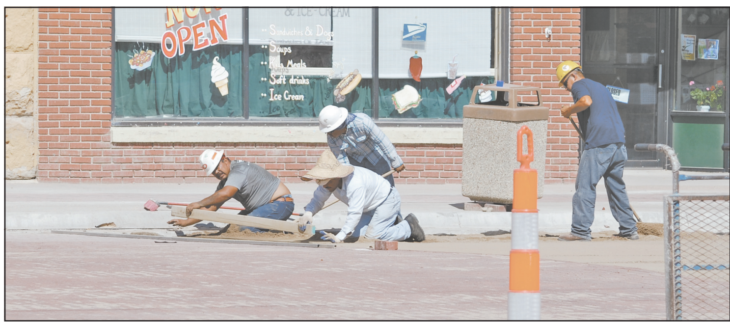
Workers began this week on laying the brick on Main Avenue between 12th and 13th Streets, signaling that the project is nearing completion and the street will soon be open. On Thursday, this crew was laying down the sand base.
