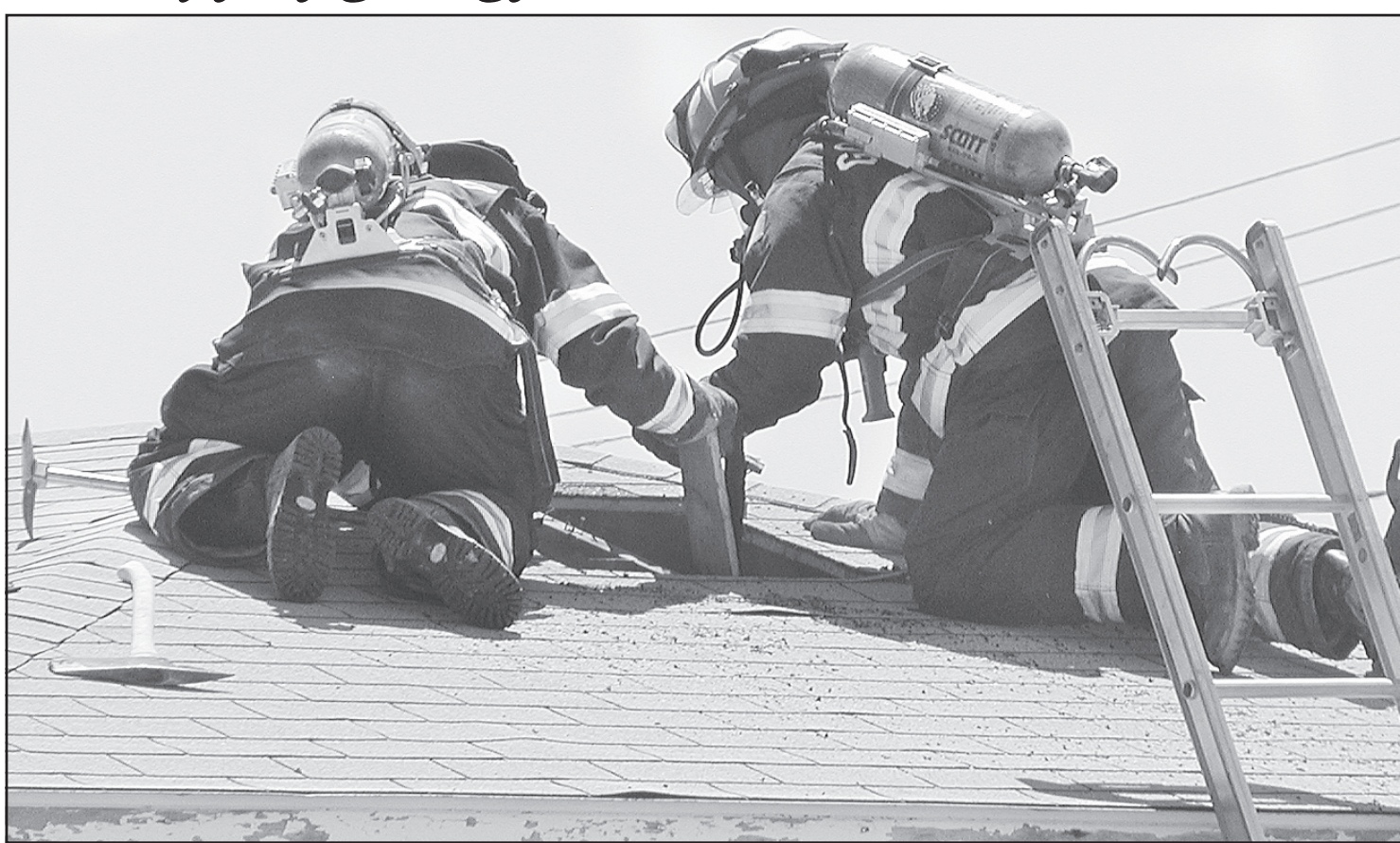
Tuesday was a hot day for fighting a fire. With temperatures at 100 degrees in the afternoon, the department responded to a small fire at Motel 7. Goodland firefighters cut a hole in the roof of one of the structures at the motel to provide some ventilation for others fighting a fire inside the building. Photo by Kevin Bottrell/The Goodland Star-News
