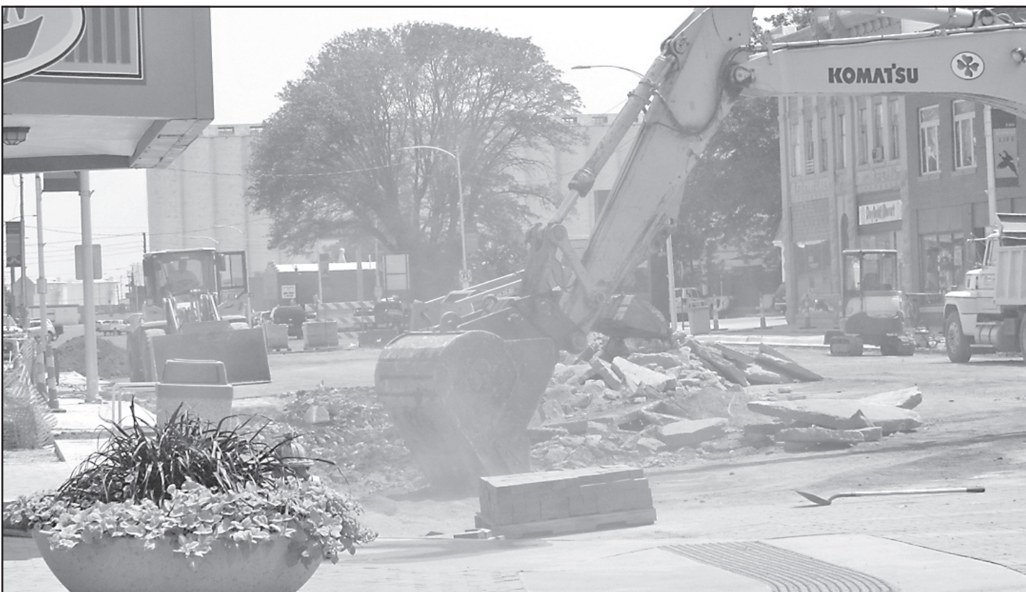
Crews were hard at work this week tearing out the old concreted one block north. The sidewalks are complete and reopened. Brick work continues Photo by Tom Betz/The Goodland Star-News
