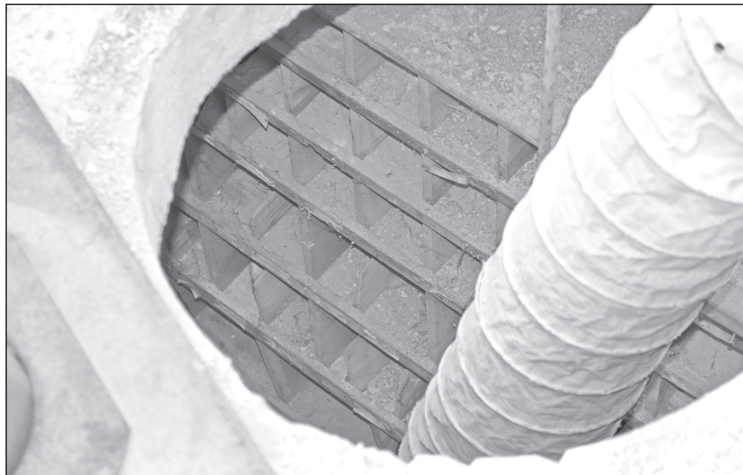
Construction crews working on the brick replacement project on Main Avenue got a bit of a surprise when they discovered this small underground room under the sidewalk in front of Olde Westport. The room was empty except for shelves. It is currently unknown
