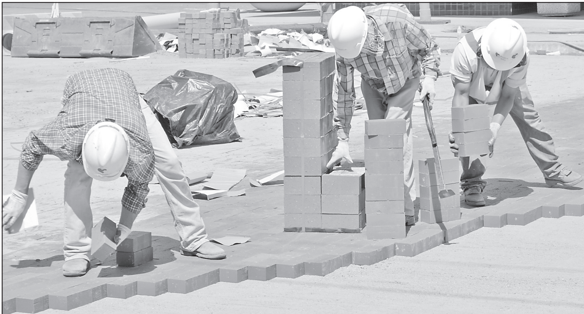
Workers began laying new brick on Main Avenue from 11th to 12th Streets early this week. The new bricks are being laid by hand in a process very similar to how original brick layer Jim Garfield Brown paved the street in 1921-1922. Photo by Pat Schiefen/The Goodland Star-News
