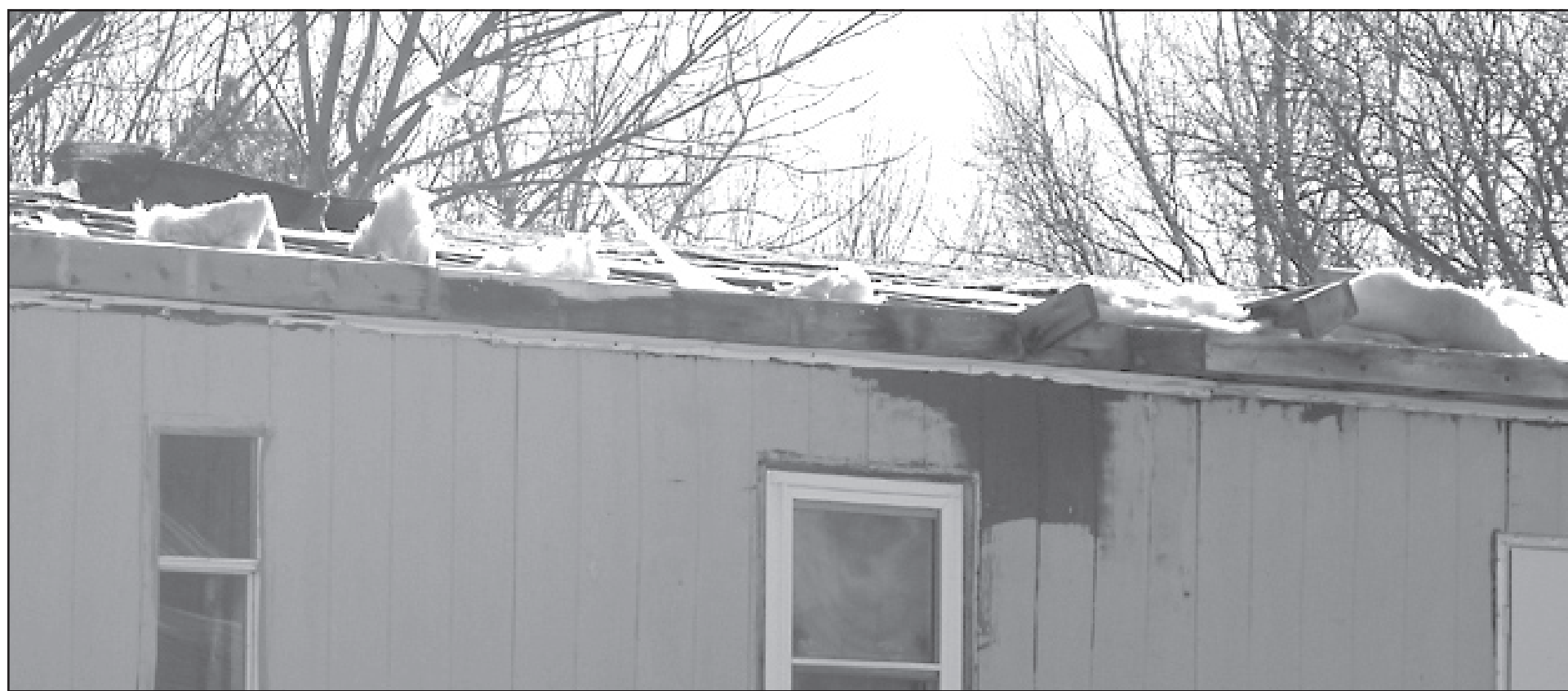
The back section of the roof of this house on Harrison Avenue was torn off by high winds Saturday. Wind gusts were measured at 77 miles per hour in Sherman County during the afternoon. The wind caused damage to homes, trees and vehicles throughout the area. Photo by Sheila Smith/The Goodland Star-News
