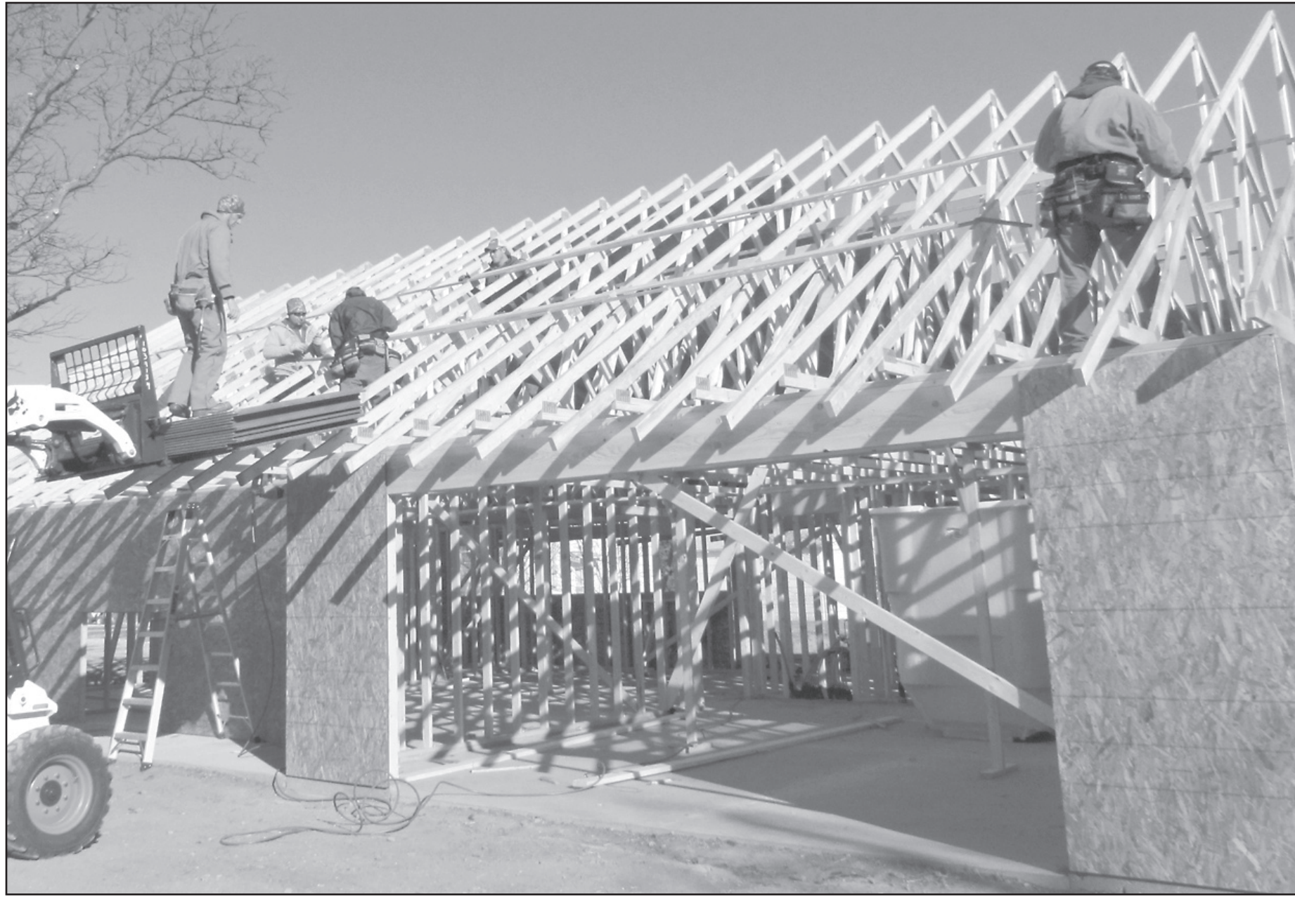
Northwest Tech Carpentry students worked hard on Thursday to get the bottom layer of roofing on the college project house at the corner of 13th and Broadway Ave. The students were hoping to beat the snow storm, but were able to get a majority of the roof on and will be working to finish this week to be able to continue
