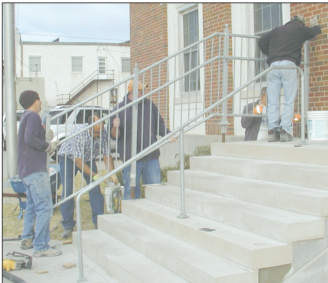
A crew of workers had to come back to Goodland last week to replace two stone slabs that cracked on the front steps of the U.S. Post Office on East 11th. The steps had been replaced earlier this year, but two developed cracks.
