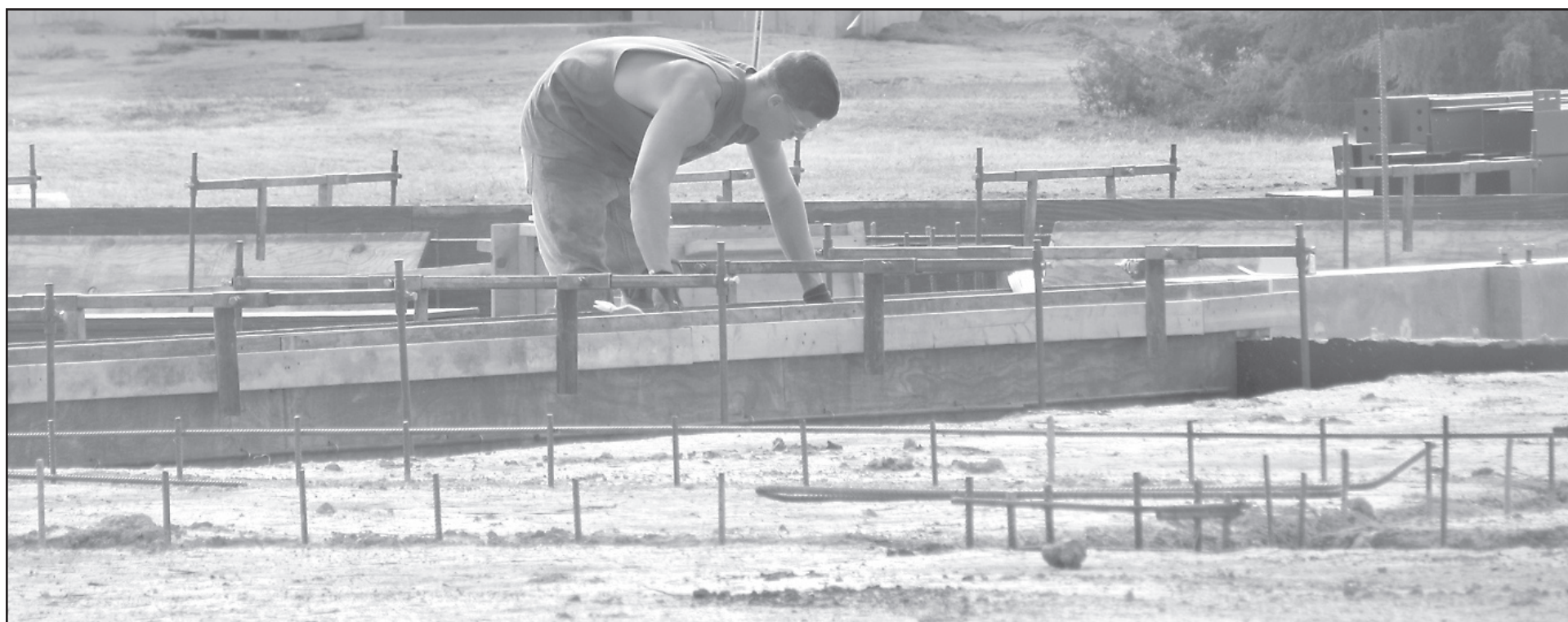
Workers are putting in forms and leveling ground for the Crop Production Services storage building in the Goodland Industrial Park west of Finley Motors. Downtown workers are beginning the process of laying the foundation for a building behind the existing Kansasland at 13th and Main.
