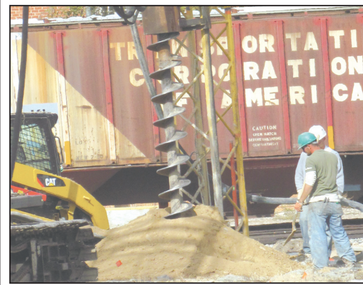
Crew from USA Tank Storage Systems of Seneca, Mo., are drilling 55-foot piers for new 500,000 gallon bolted tanks to be erected for Agro Culture Liquid Fertilizer south of the railroad tracks. Each tank will take 63 piers before the slabs are poured. A spokesperson said they hope to have the slabs ready in November, and ready for the tanks to arrive.
