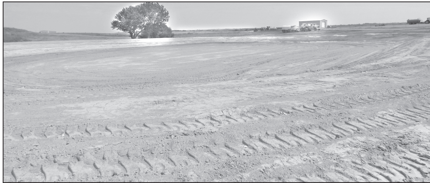
City Public Works Director Rich Simon said Tuesday the temporary sewer pond is about ready, and he hopes to have the pipe delivered on Monday so the project to drain and clean out the existing pond can begin later in the week. He expects the project to be done by early October.
