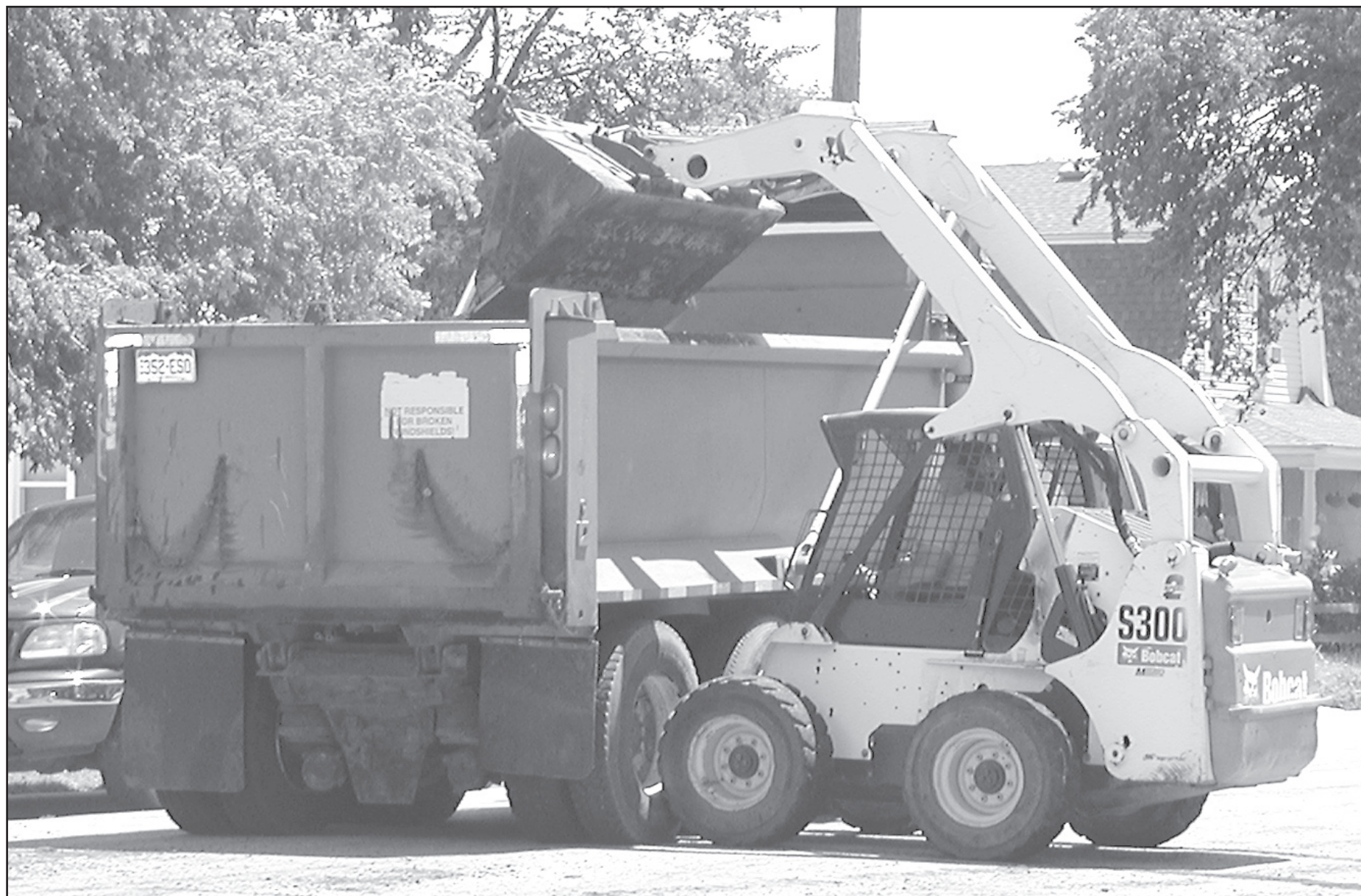
APAC of Hays started the mill and overlay work on Caldwell Tuesday morning. The overlay was to run south of 8th Street and past the intersection of 10th and Caldwell. Workers had to work around pipe work before the intersection of 10th
