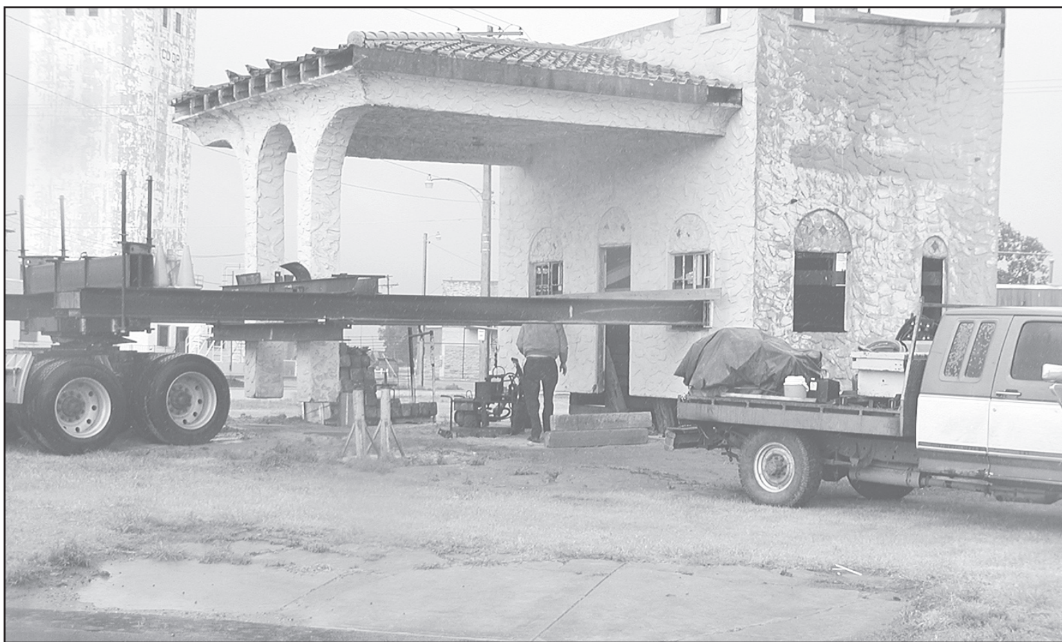
The moving company hired by Rod Cooper to move a historic gas station from Kanorado to Goodland were working to get the building set down.
