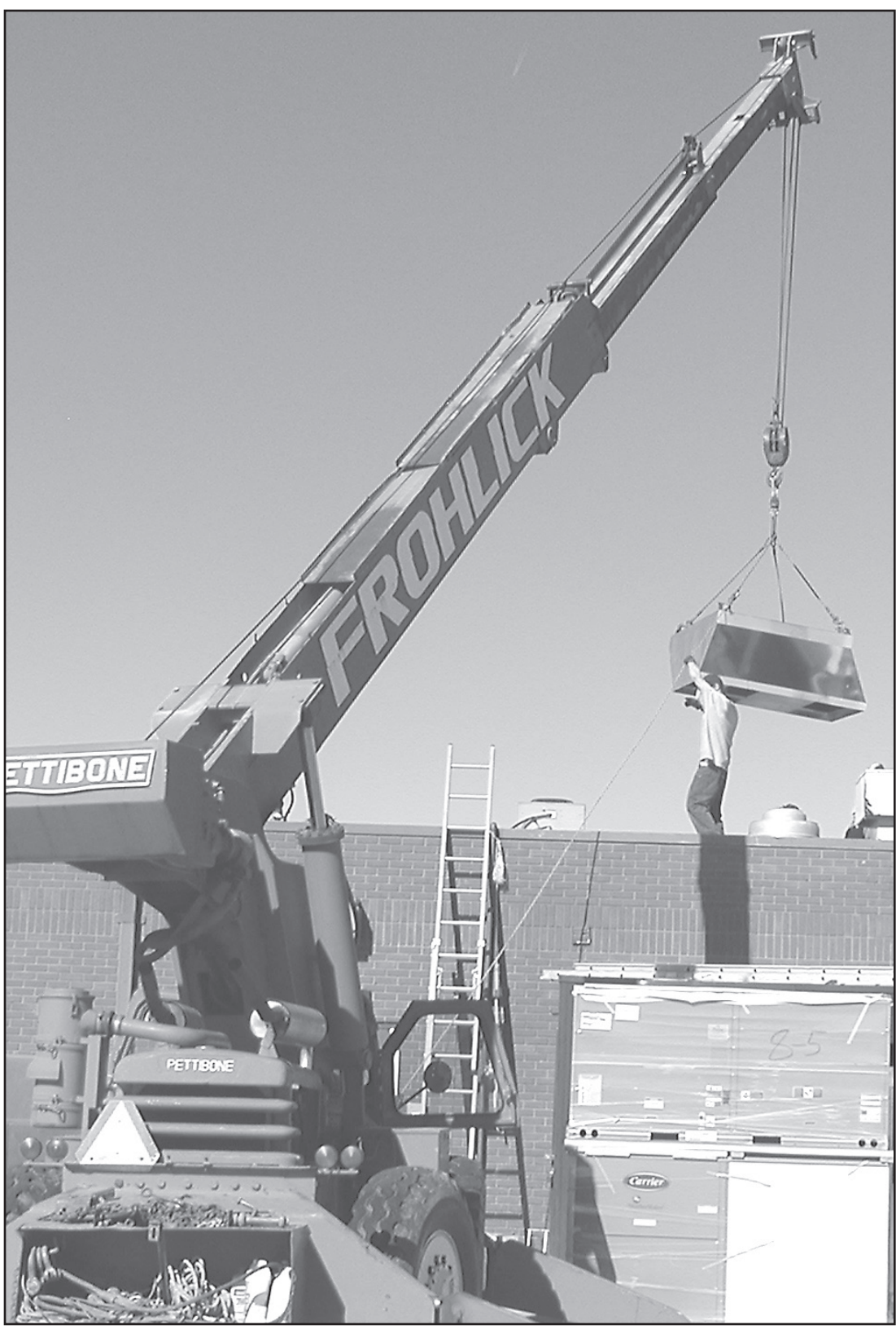
Subcontractor Burlington Heating and Air Conditioning for McClure's Plumbing and Heating of Colby brought in a crane to lift new air conditioning and heating units at Wendy's, 2219 Enterprise Road. The weather and wind cooperated for the work to be done on Tuesday morning. Photo by Pat Schiefen/The Goodland Star-News
