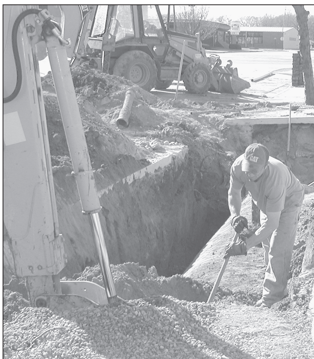
Employees of VanKirk working on the Goodland water project were running water lines and ran into a buried tank under the sidewalk at the Centennial Building at 10th and Main. They were going to remove the tank.
