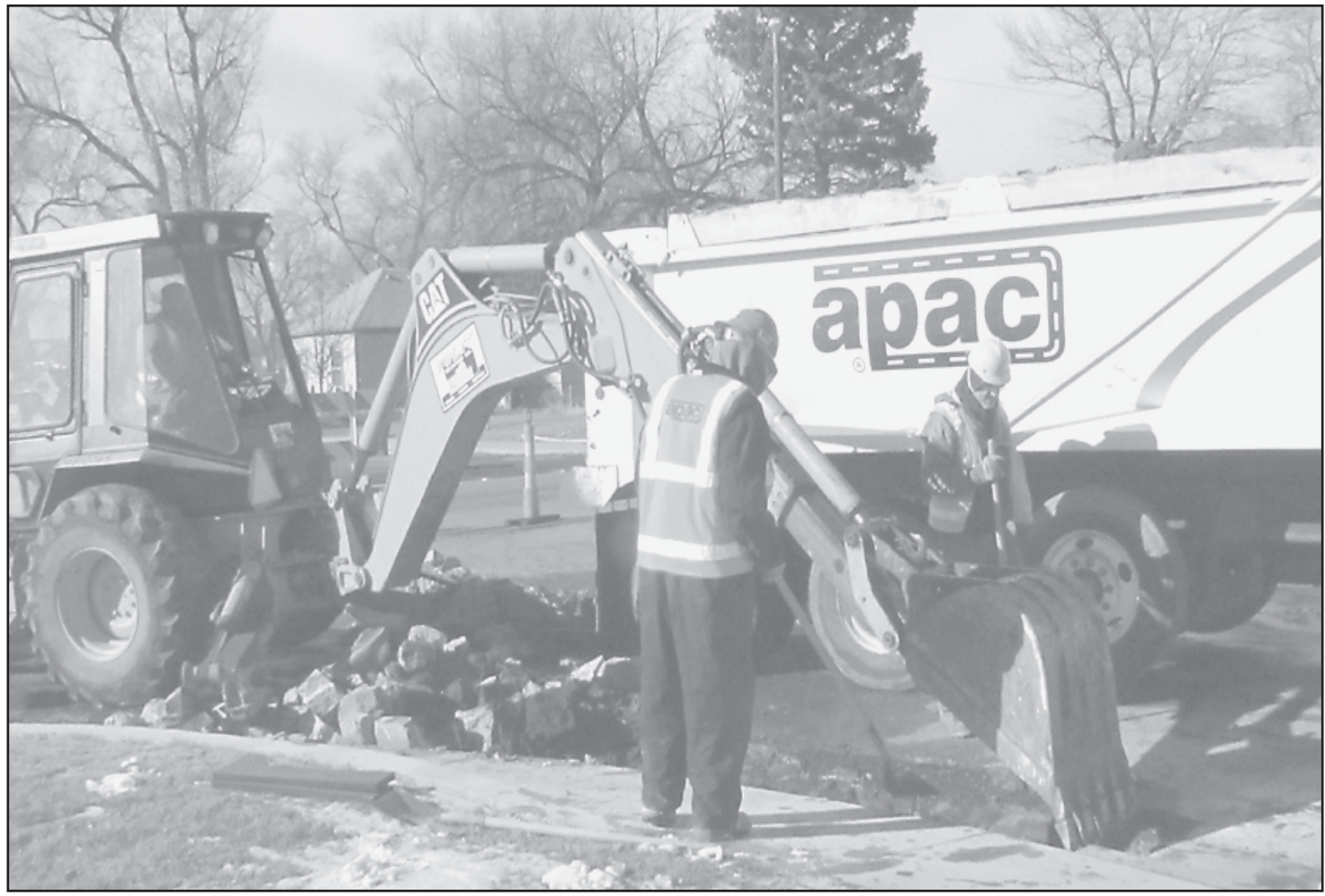
A crew from APAC of Hays is starting the new year working on the corner and valley gutter at 11th and Caldwell Ave. The work will continue through the spring as APAC gets the curb and gutter and valley gutters along Caldwell ready for the next step a mill and overlay to be done in the spring. Photo by Tom Betz/The Goodland Star-News
