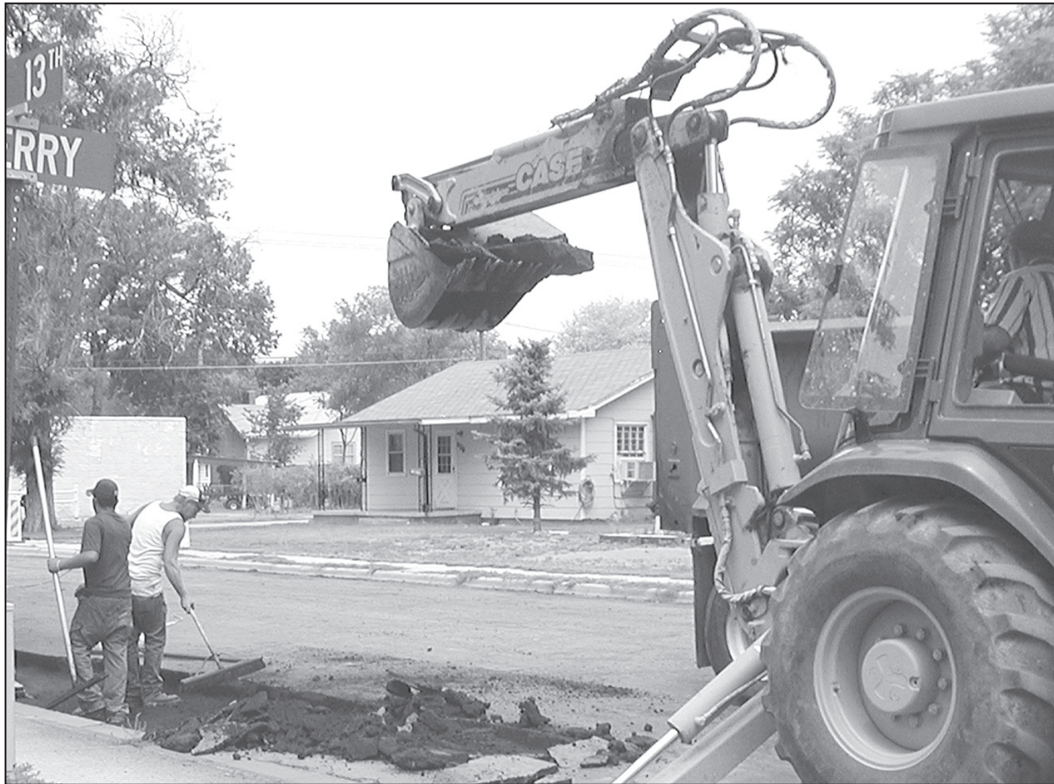
Workers for Glasser Construction of Stratton, Colo., were tearing up asphalt at 13th and Cherry on Tuesday to get it ready for new. Photo by Pat Schiefen/The Goodland Star-News
