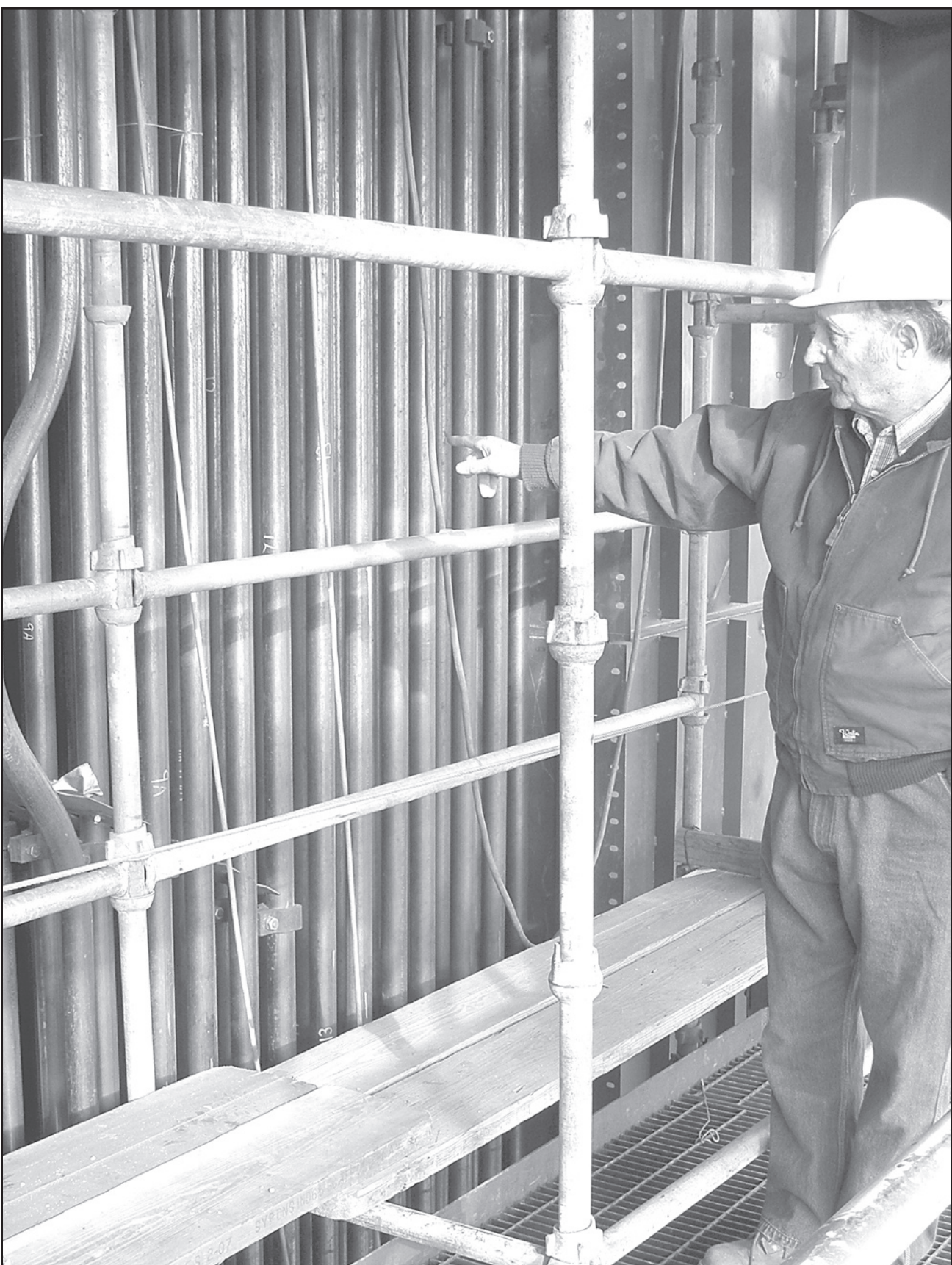
Norman House, president of Goodland Energy Resources, the partnership building a power plant five miles west of Goodland pointed out the rows of the hundreds of new boiler tubes that have been installed and inspected as part of the construction during a tour of the plant on Friday.
