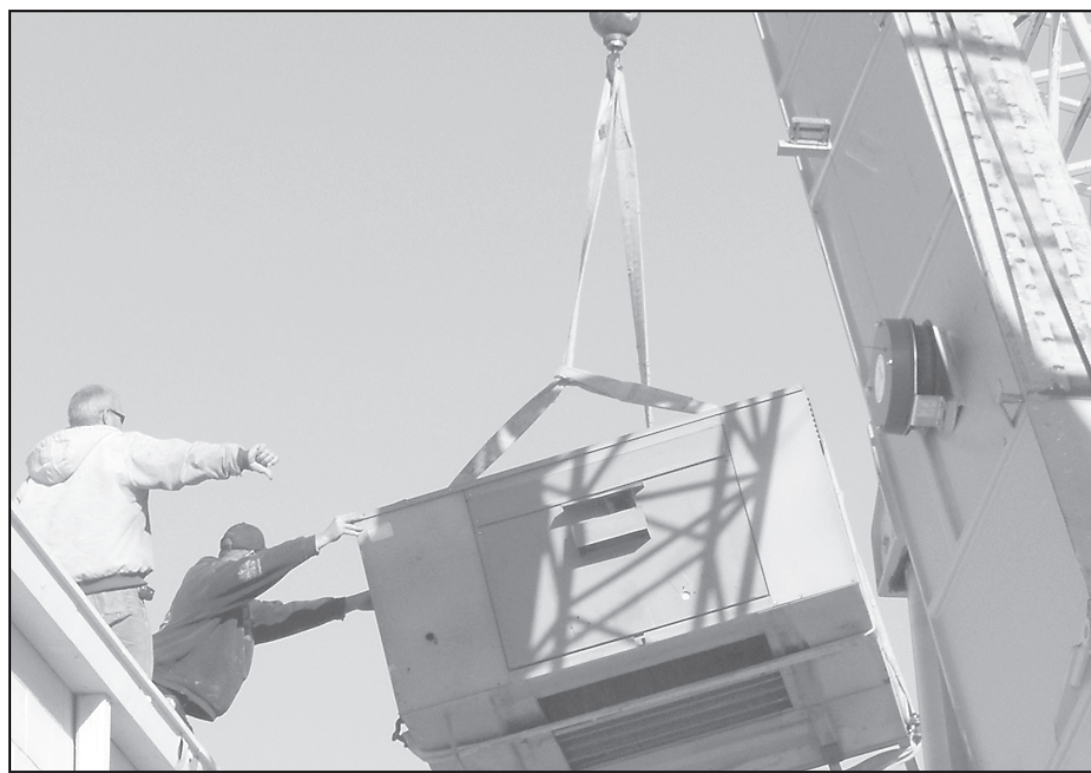
Workers from Colby-based Woofter Construction installed a heating and air conditioning unit Friday at First Baptist Church on Main Street.
