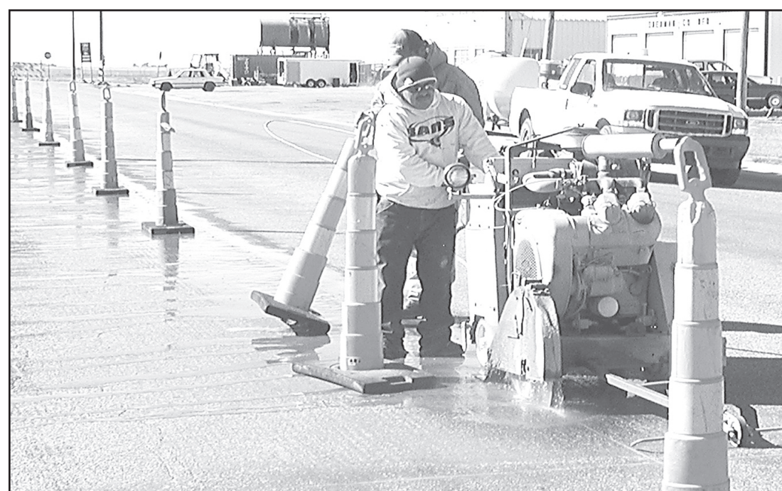
Juan M. Gonzalez, a worker for Oakley-based Sporer Land Development Inc., operated a large saw to cut concrete on Monday near the corner of Eighth Street and D’Lao Drive in Goodland as worker Ignacio Ramirez assisted. The street was being cut so new concrete can be laid, Gonzalez said. Photo by Ramona C. Sanders/The Goodland Star-News
