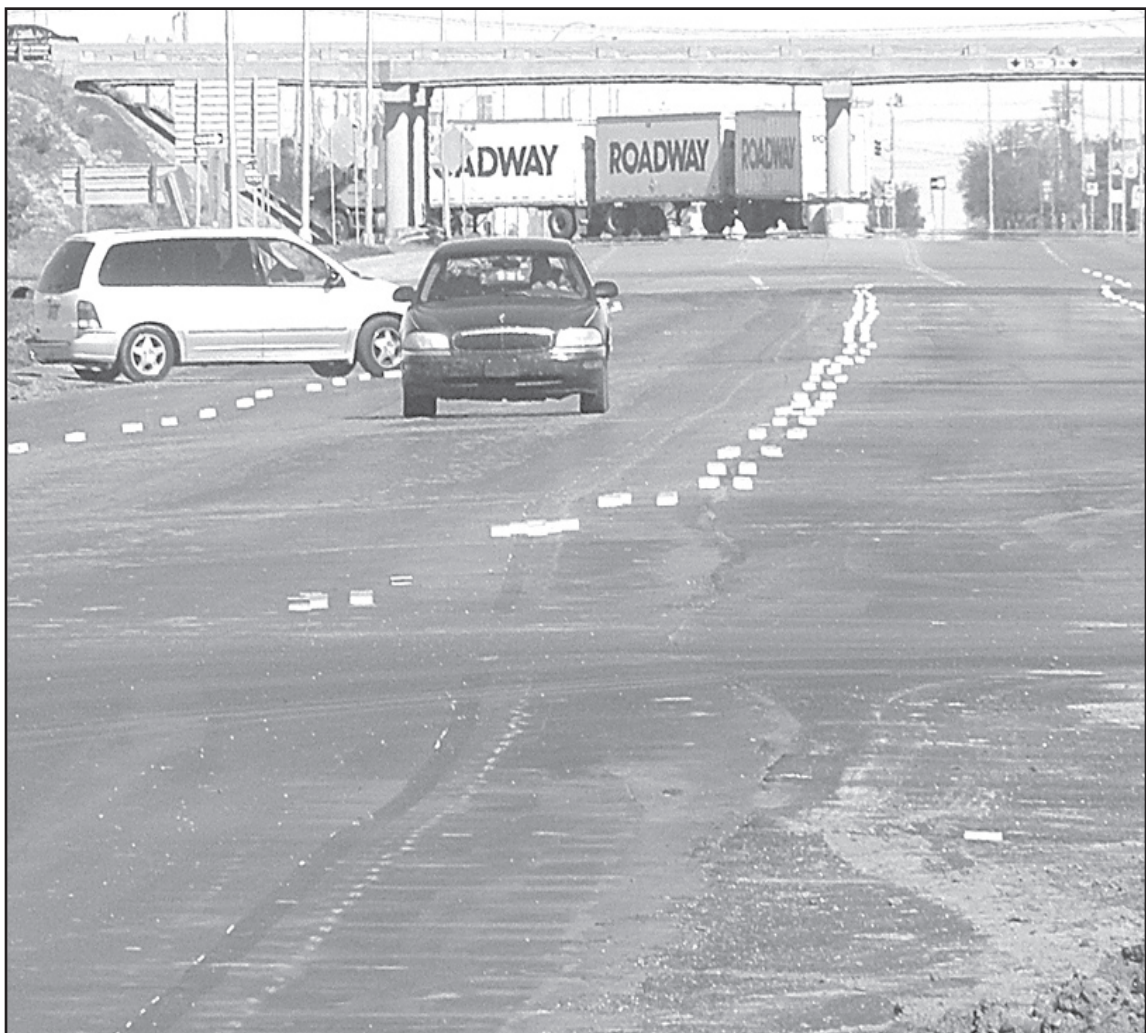
Paving has been completed on the north end of the new K-27 road south of town. Permanent striping and finishing work will continue over the next month, state highway department Contract Engineer Michael Terry said.
