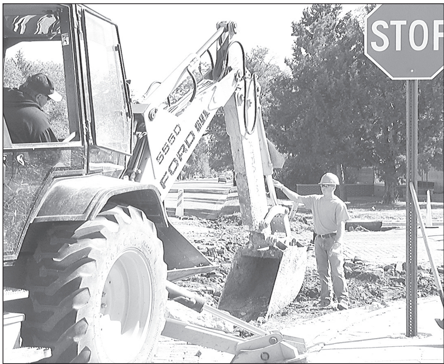
City worker Justin Lohr gestured to coworkers Tuesday as they began demolishing and replacing the valley gutters at 12th Street and Broadway. The work includes installing a new fire hydrant on the southeast corner of the intersection, Lohr said.
