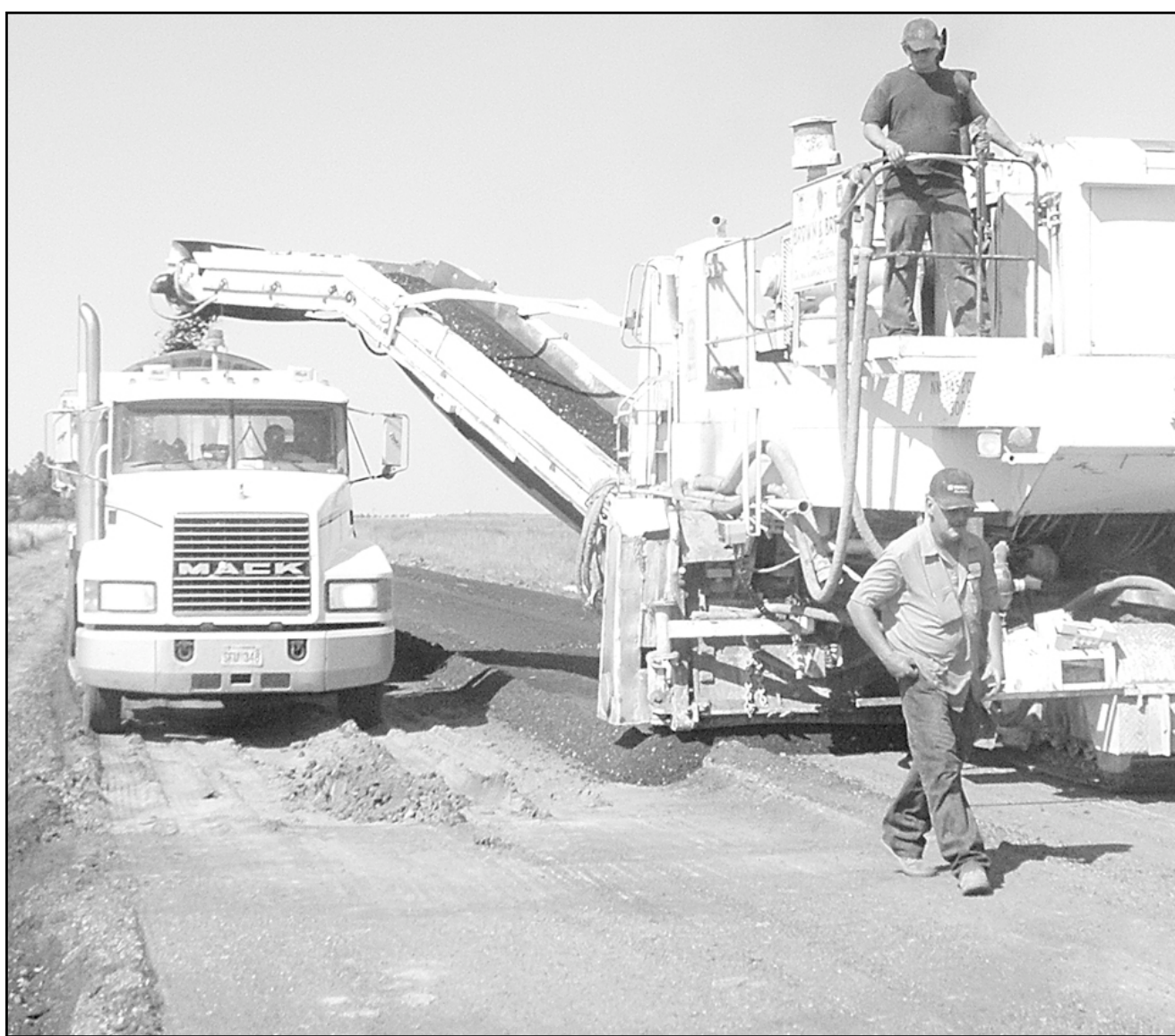
Crews from Brown and Brown of Salina ripped out the old section of K-27 south of town on Wednesday as the project to build a new roadway to the east winds up with the opening of the road from south of the Smoky Hill River to the Sherman County line. Photo by Tom Betz/The Goodland Star-News
