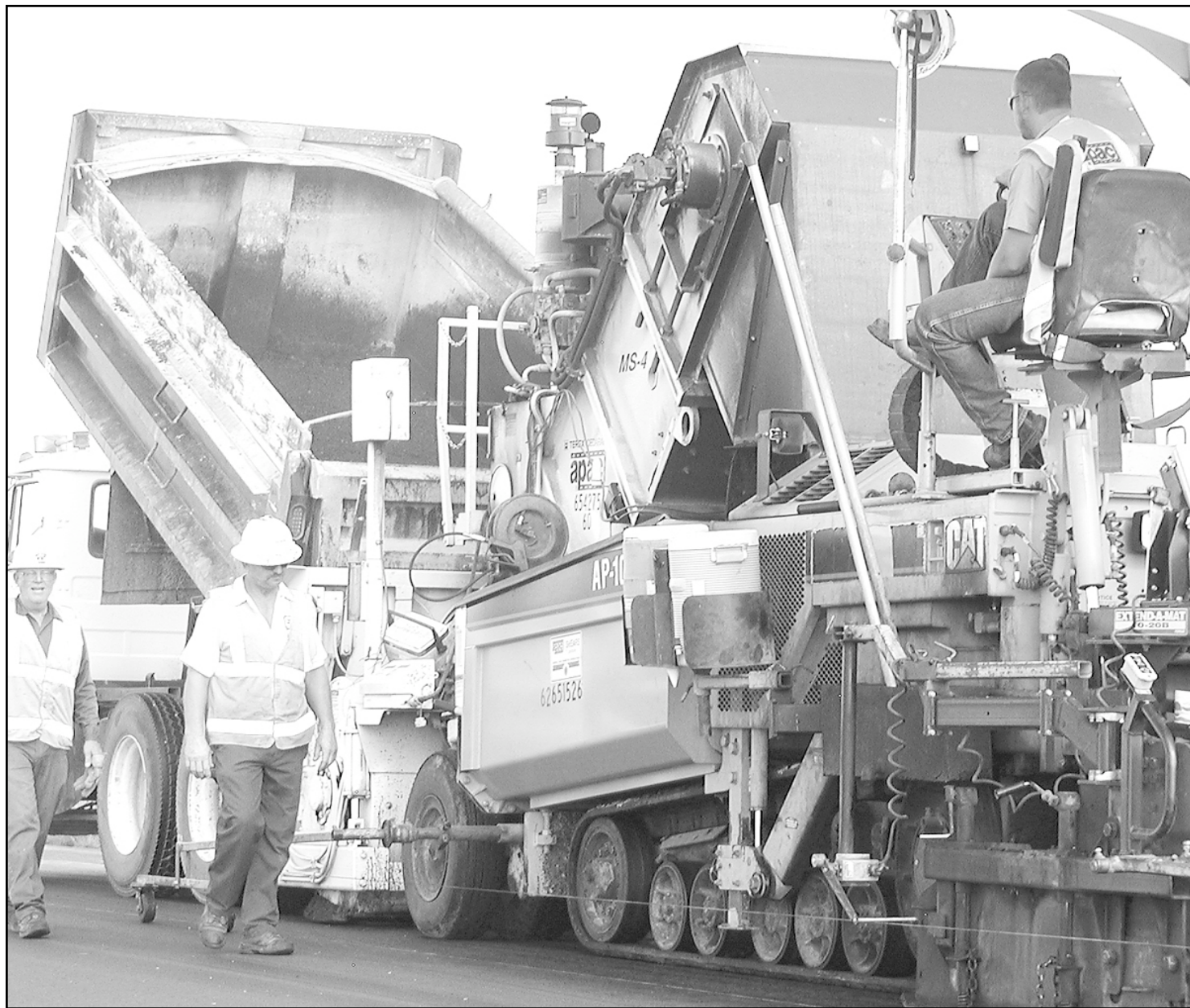
Crews from APAC Shears of Hays were paving on old U.S. 24 about four miles west of Caruso on Friday, working their way east to Goodland. The old U.S. 24 project is the largest of the county road projects being paid for through the special one-cent sales tax. Darin Neufeld, engineer for Evans, Bierly, Hutchison and
