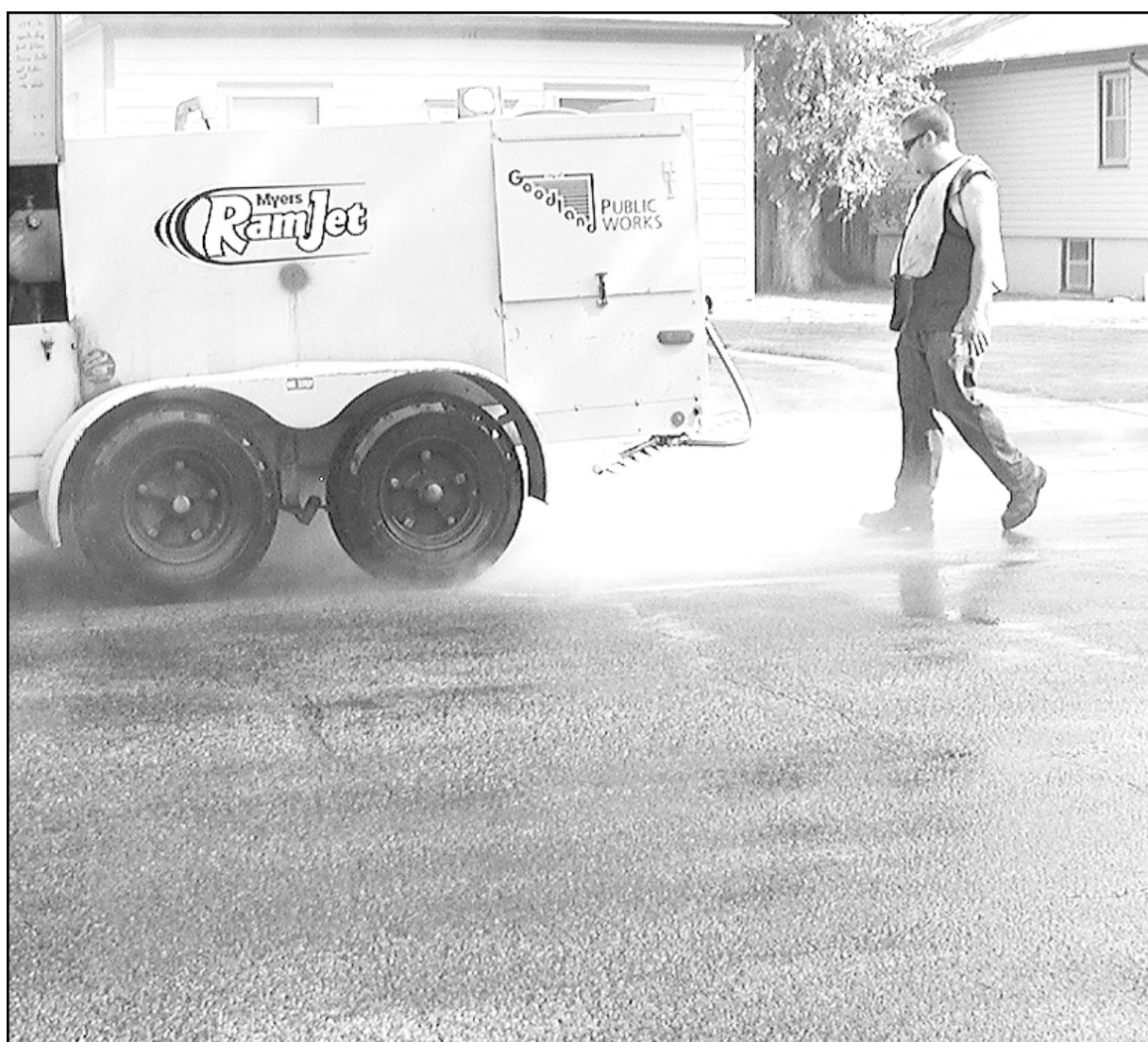
City crews washed 10th Street on Friday in anticipation of a sealing project which was to begin this week. Phil Erickson, street department superintendent, said Monday the contractor had been delayed, but the sealing should begin next Monday and take about three days.
