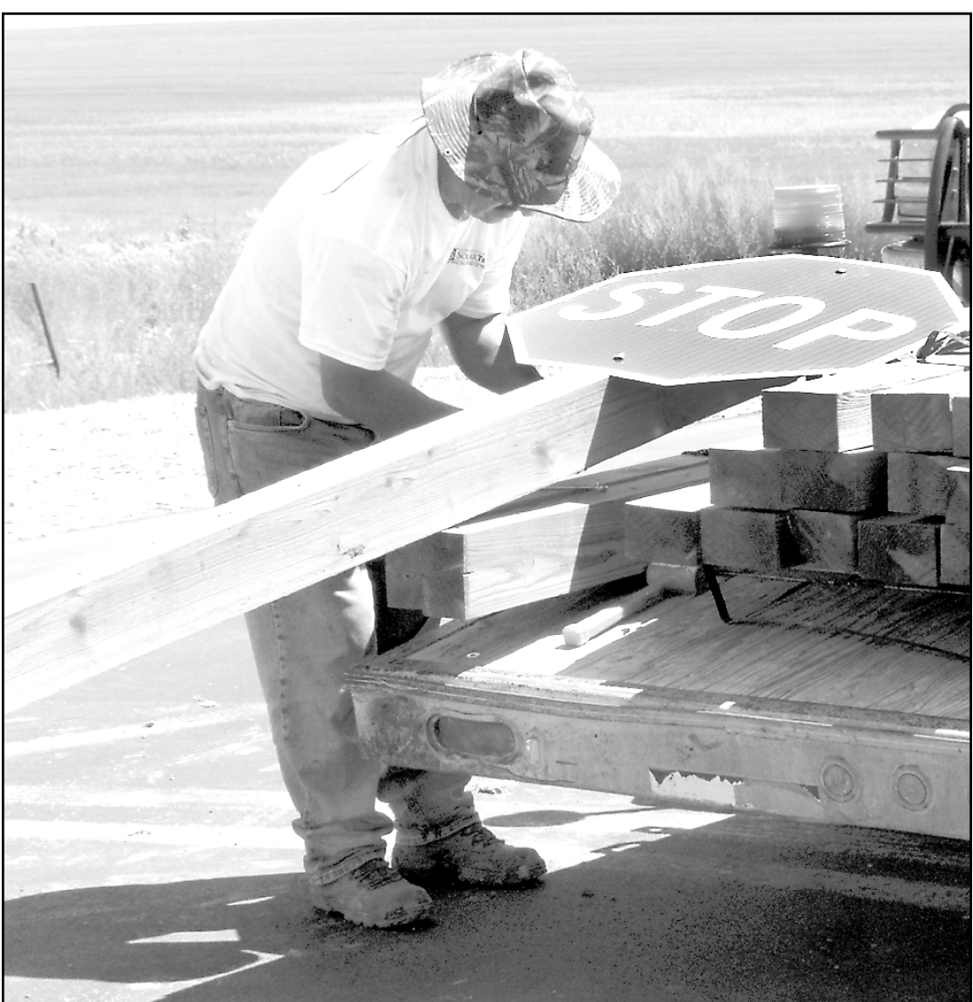
Jose Avalos-Robledo of Cillesten and Sons of Wichita was busy Wednesday afternoon attaching signs to posts to be set along the new stretch of K-27 about a mile south of town that should open for traffic on Monday. Manuel Villareal-Perez was cleaning out the post holes drilled by another crew member with a small tractor. Photo by Tom Betz/The Goodland Star-News
