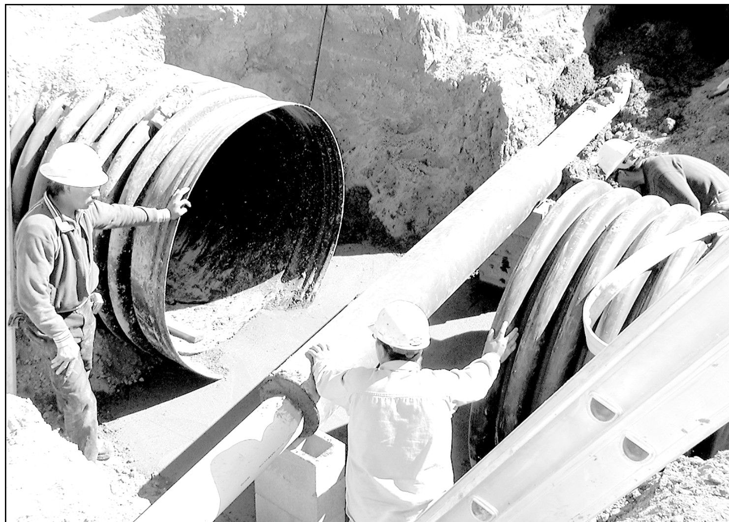
Sections of the new storm sewer on the south side of 17th Street were being put in place on Monday as the construction project moved ahead. The crews from Midland, a sub-contractor of Sporer Land Development, were moving quickly to get the storm sewer installed. The cone zone has 17th down to one-way traffic from Cherry to Broadway, and the project will go all the way to Main. The project is being paid for by the special one-cent sales tax that went into effect in July. The city project on Caldwell is ready to start, and more cone zones will appear as work progresses.
