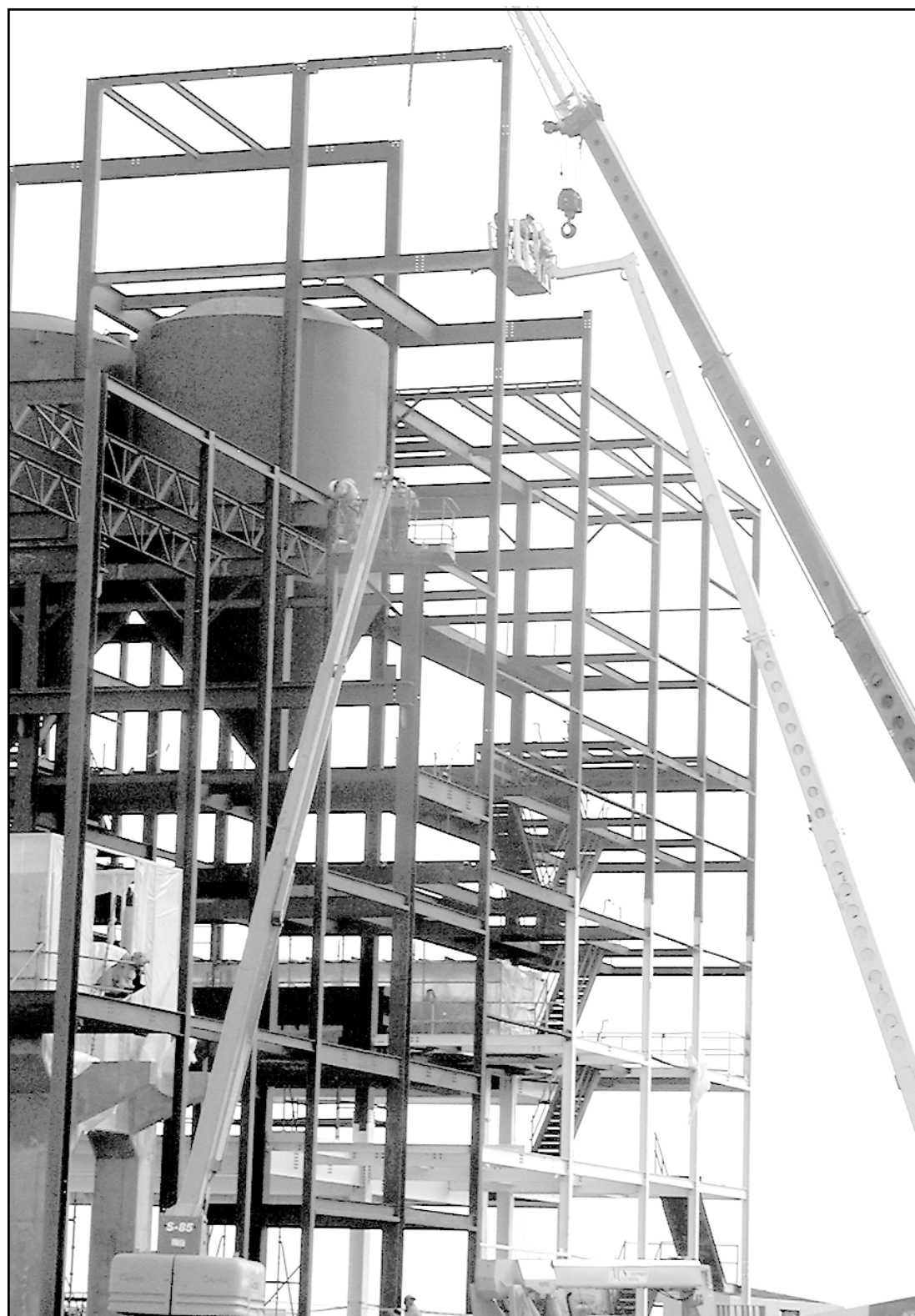
Workers reached high into the steel on powered lifts at the coal-fired power plant at the Goodland Energy Center on Wednesday. The coal bunkers didn't seem as large once they were lifted into place. Work has begun on the surrounding structure to assemble the other parts of the plant and enclose the building.
